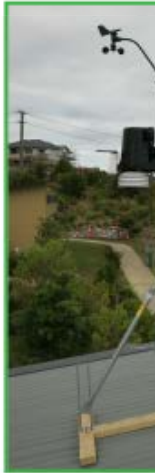
AIR TEMPERATURE, RELATIVE HUMIDITY, WIND SPEED AND DIRECTION MONITORING ON ROOF
