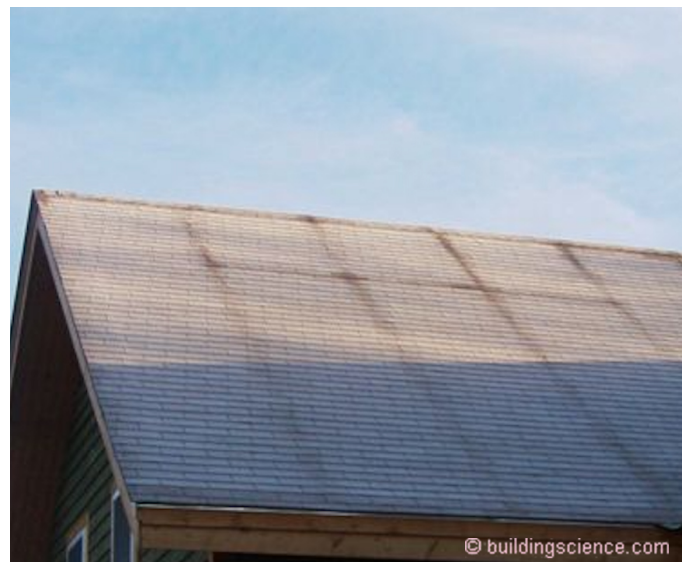
Photograph 2: "Telegraphing" of panel joints in roof assemblies under asphalt shingles.
