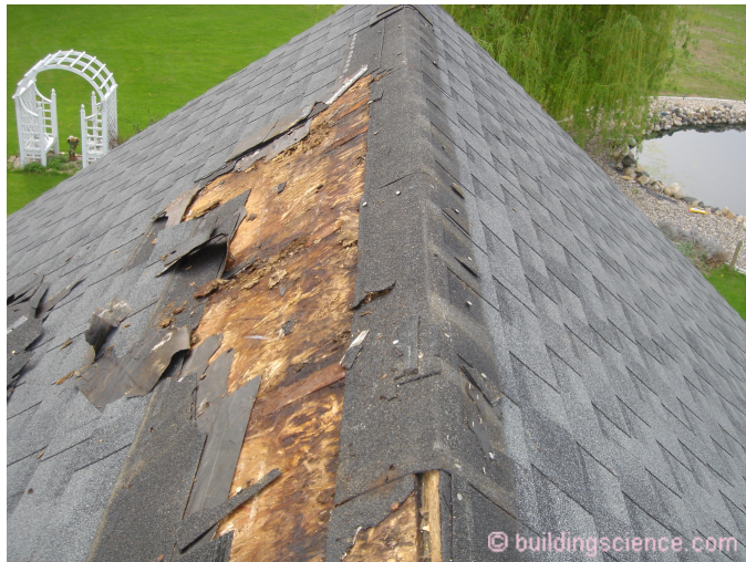
Photograph 1: Bad stuff happens at ridges...."ridge rot".
