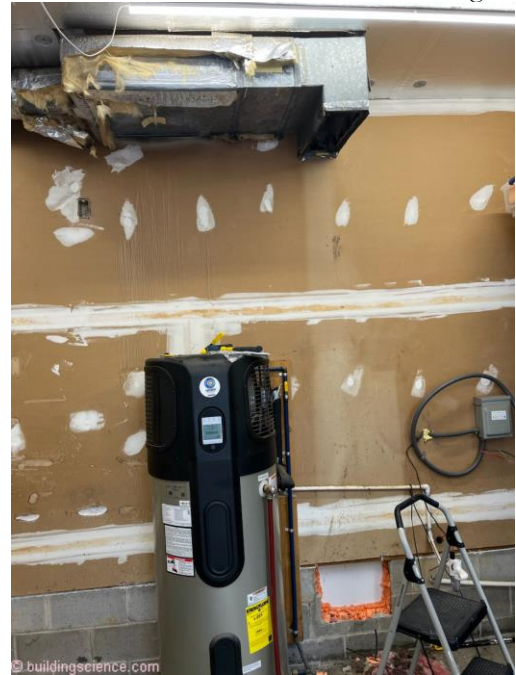
Photograph 2 from Alex DeSpain. HPWH Garage Installation. The outline of the now missing air handler unit is visible on the dry wall. Cold air discharge pointed directly at air handler. High dew point temps in garage near Richmond, VA. Condensation on air handler and supply ductwork caused mold. Equipment was removed.
