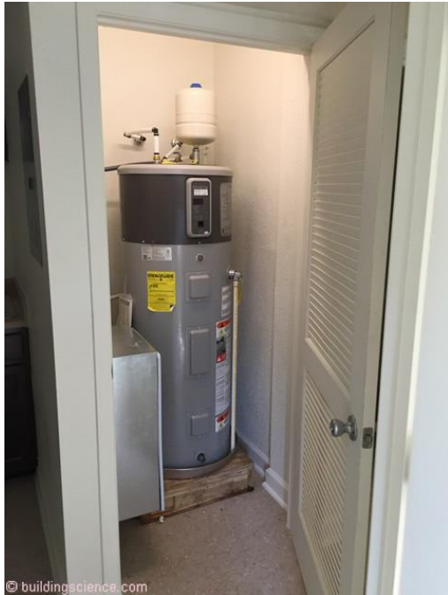
Photograph 1 from Nikki Krueger. HPWH Closet Installation. Cold air discharge impacts back wall. Full louvered door allows gravity convection air exchange. However, incoming air has high humidity/dew point.
