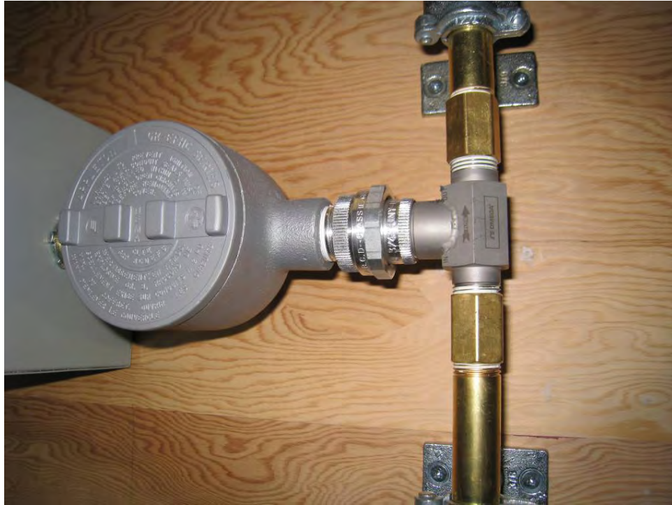
Figure 27 – Cooling Water Flow Meter (right) and Signal Conditioner (left)
