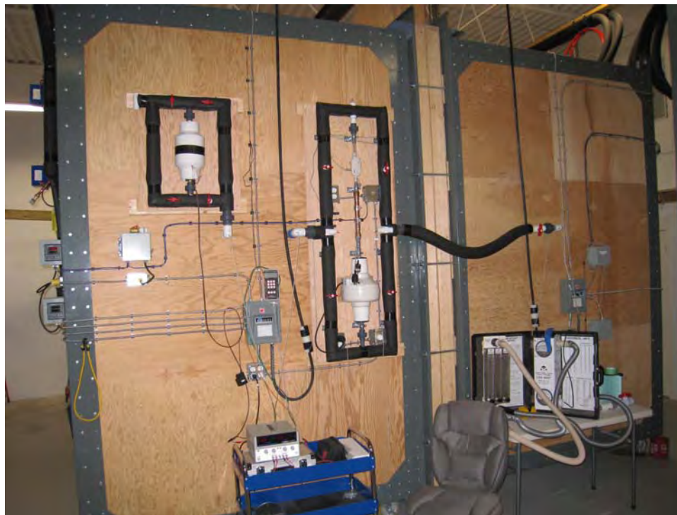
Figure 8 – Guard Fan (Left) & Air Transfer System (Center)
