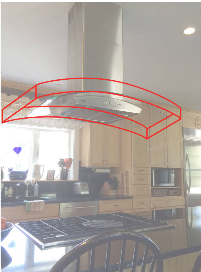
Photograph 2: Kitchen Range Hoods - We are getting better capture efficiency with better hood design and that means we can get away with lower exhaust flows.
