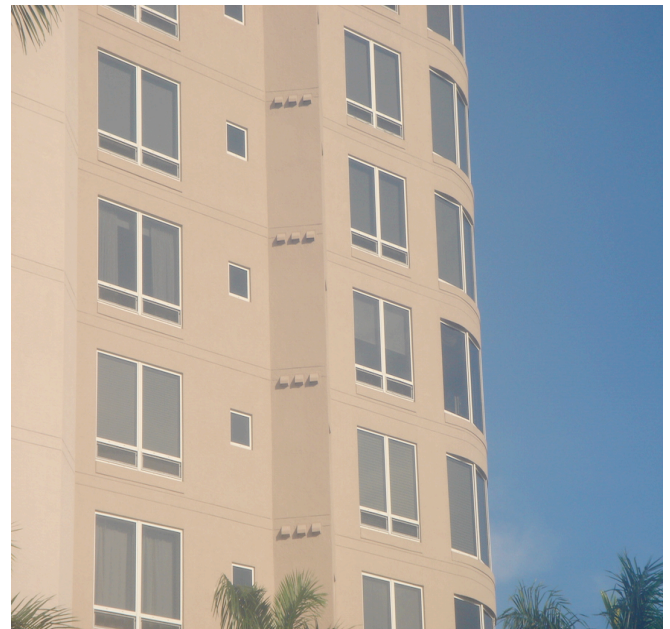
Photograph 4: Lots of Penetrations - You want energy efficiency? You want a controlled indoor environment? You want to build tight and ventilate right? You better get used to living with the holes. Putting the stuff on the roof or at the bottom of the building does not work. Might work in houses and row houses and town houses but not in apartments.
