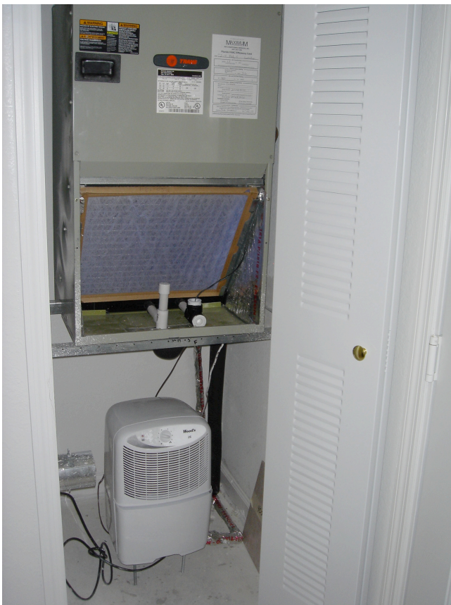
Photograph 1: Dehumidifier In Return Closet – Works but we can do better.
