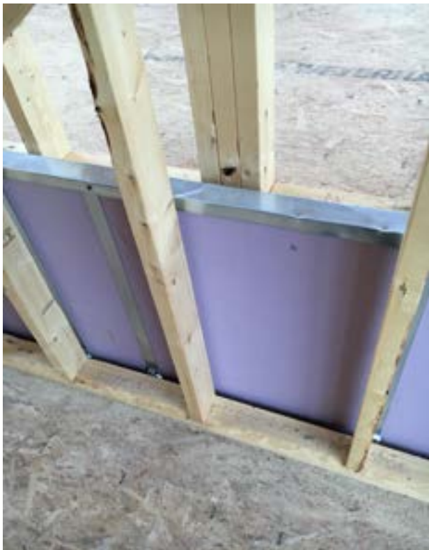
Photograph 4: Fire Wall - The most common fire wall is two (2) one inch (1”) layers of gypsum board in an “H-Stud” channel and runner system with aluminum breakaway clips. Regular wood frame walls get constructed on each side with a ¾ inch continuous air gap between them and the gypsum boards. This is a beautiful thing. Fast to construct. Practical. Works. All good so far. But air leaks along the gaps – upwards and sideways and inwards and outwards and every which way. Ugh! Got to stop that airflow.
