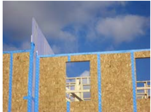
Photograph 10: Membrane Strips – No so ugly after all. Note the membrane strip over the top of the front of the wall – check out Figure 7 for the rationale.
