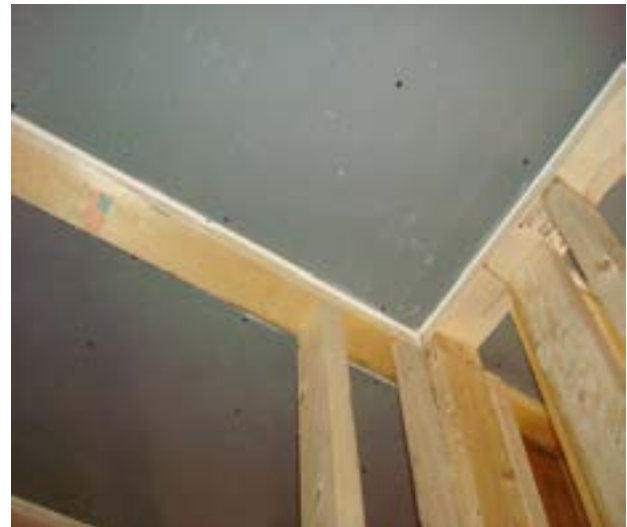
Photograph 6: Sealing The Lid - We need the "lid" at the roof-ceiling interface to be airtight as well. This involves the gypsum board ceiling. The boarders install the gypsum "lid" first – and before they install the wall gypsum board and then a "fillet" bead of sealant is installed at the perimeter of every room at the ceiling line providing an airtight seal between the ceiling gypsum board and the top plates of the wall framing on both interior and exterior walls and the fire wall framing.
