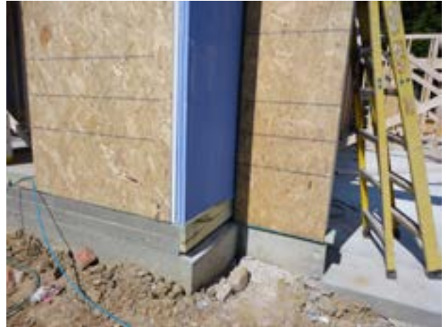
Photograph 7: Off-Set Adjacent Units – Note the protruding gypsum fire wall.
