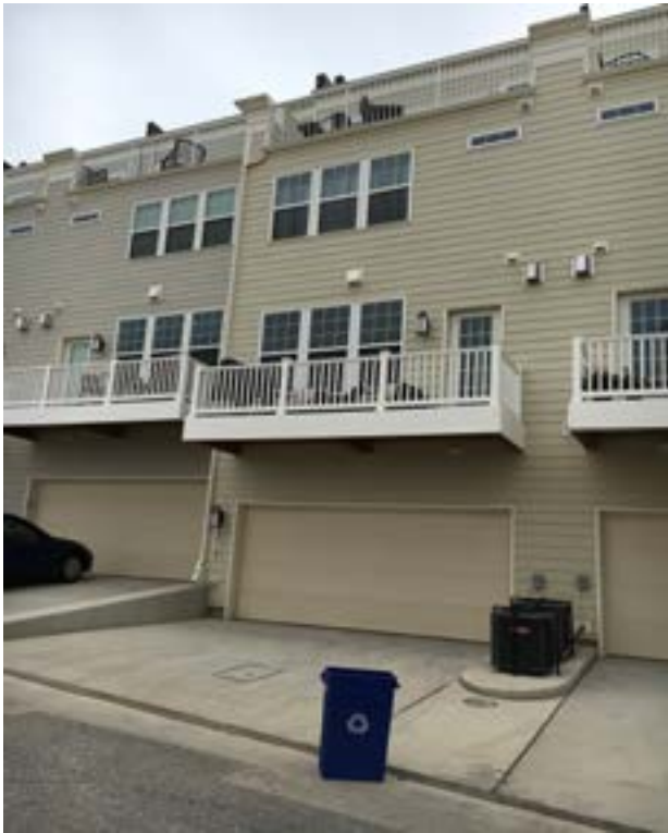
Photograph 2: Tuck In Garage – Living space over a “tuck-in” garage is a nightmare to seal around a fire wall in a townhouse or row house.
