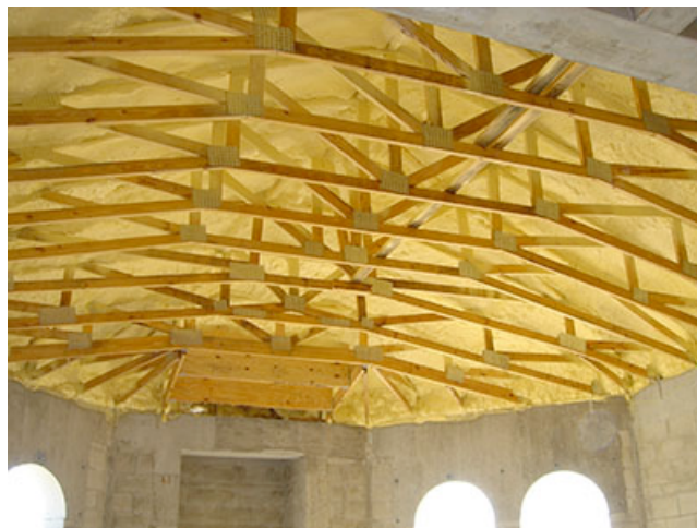
Photograph 2: More Open Cell Low Density Spray Foam - Moisture in the indoor air migrates into the attic spaces, passes through the open cell low density spray foam and is stored in the wood based roof sheathing. It then gets driven out by temperature changes – largely driven by solar radiation – and accumulates at the upper portions of attics.
