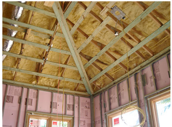
Photograph 1: Florida Open Cell Low Density Spray Foam - The key to understanding what is going on is the storage capability of the wood based roof sheathing and the permeance of the spray foam. Open cell low density spray foam is very vapor open – around 30 perms per inch of thickness – and will allow moisture from the interior air to pass through it and migrate to the underside of the roof deck – the wood based roof sheathing.
