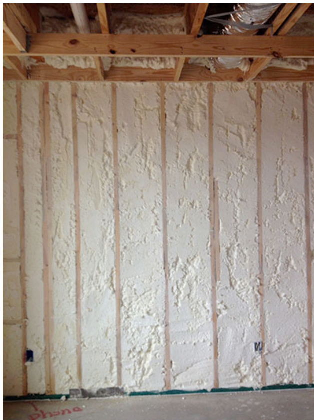
Photograph 4: Open Cell Low Density Spray Foam in Walls – We do not see these issues with open cell low density spray foam used in walls. In a typical house, the roof area is large with high exposure to solar gain and night sky radiation with minimal vapor control separation to the interior space. These are not major factors with walls and note that walls are typically covered with painted gypsum board – a pretty good vapor “throttle”.
