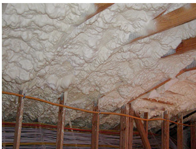
Photograph 3: Cold Climate Open Cell Low Density Spray Foam - “Leaky ductwork” did not solve the problem in cold climates with no attic ductwork. Only vapor retarder coatings coupled with some form of air change via a fan solved the problem in cold climates. The code requires a vapor retarder on open cell low density spray foam in IECC Climate Zones 5 and higher – but it is typically ignored by installers – and shame on them. And the manufacturers do not police the installers – and shame on them too. And the building officials that let them get away with it. Where is Aretha Franklin when you need her....“shame, shame, shame....”
