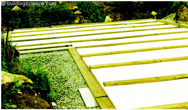
Photograph 9: Wood-Slab-On-Grade Foundation - Start with a gravel pad, lay out your membrane water control layer, air control layer and vapor control layer, lay out your perimeter wood footing and lay down your continuous rigid insulation. Note the concrete “pad” that provides support for a “point” load.
