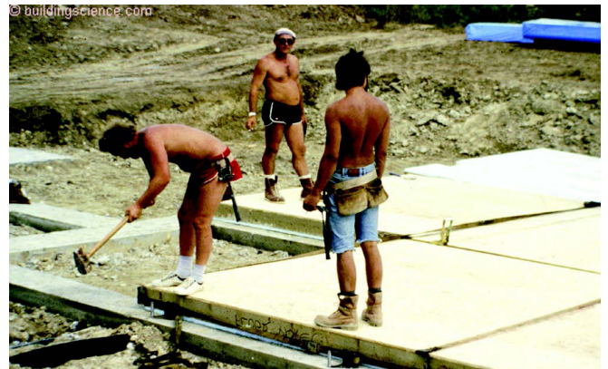
Photograph 6: Panelized Wood Basement Floor Slab – Panels supported on concrete footings. Note the extruded polystyrene rigid insulation on the bottom side of the panels. It was tough to get the gaskets to air seal the panel joints.
