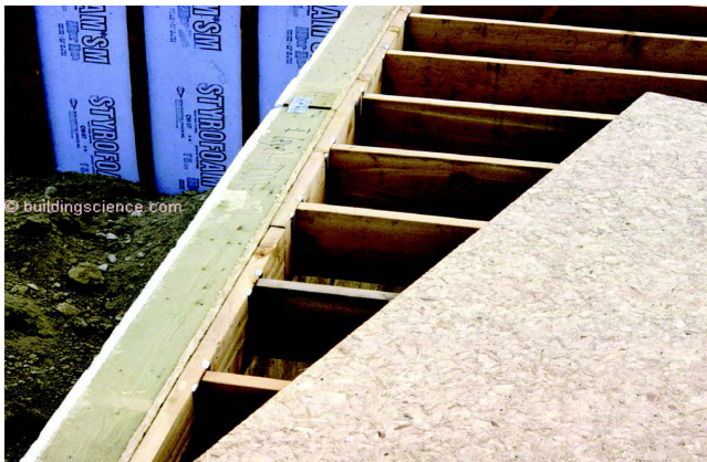
Photograph 8: “Balloon Framed Foundation” - Note how the main floor is framed below the top of the perimeter wall to handle the “back-fill” load.
