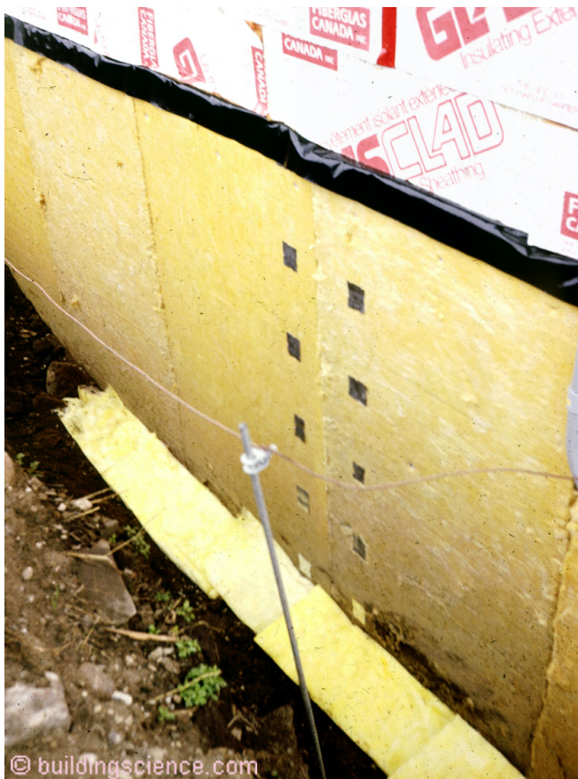
Photograph 2: Fiberglass Roofing Insulation - In Canada I couldn't get rigid fiberglass stuff that was to be used below grade, so I used fiberglass insulation boards typically used in commercial flat roofs. Notice the metal plates on the exterior of the fiberglass – they are “compression” measurement plates. I wanted to know how much the insulation would compress over time. I could read them from the inside using a linear gage...called a nail.
