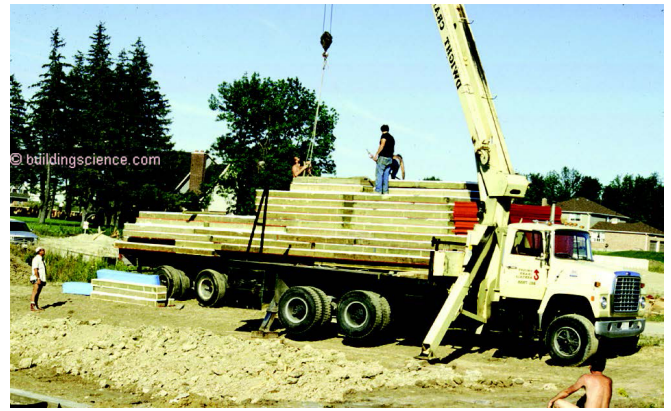
Photograph 5: Panelized Wood Basement Foundations - I played around with panelizing the wood basement foundations...yes, I started my own panel business...lost a lot of money.... have strong opinions on panelization.
