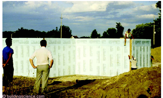
Photograph 7: Panelized Wood Basement Foundation Walls – It was tough to get sealants or gaskets to function as reliable 2-stage joints to control water leakage and air leakage at panel joints.
