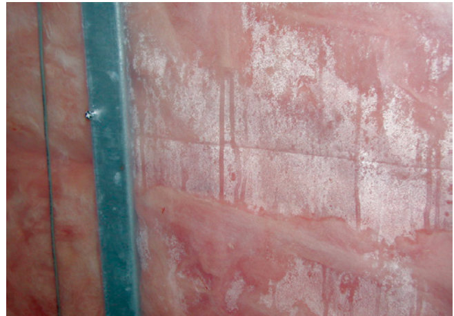
Photograph 9: Condensation on Polyethylene Vapor Barriers —Solar driven moisture out of reservoir claddings can lead to cavity side condensation on polyethylene vapor barriers in cold climates such as Chicago.
