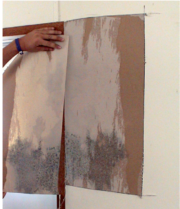
Photograph 6: Vinyl Covered Gypsum Board —FEMA trailers are lined with vinyl-covered gypsum board as are HUD manufactured houses. This leads to mold problems. The only solution is to not install vinyl covered gypsum board.
