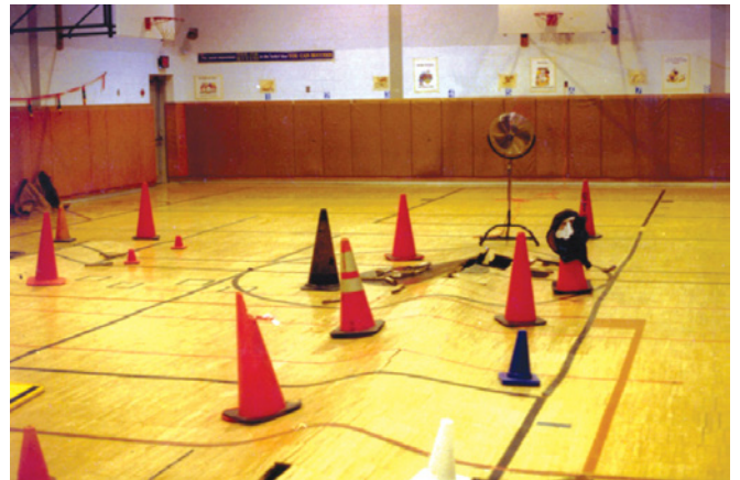
Photograph 2: Buckling Wood Floor —If wood is not conditioned to the mid point of its expected moisture content range prior to installation it will buckle.
