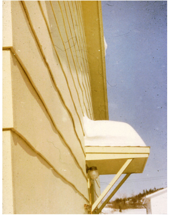
Photograph 1: Buckling of Hardboard Siding —Hardboard grows along its length as relative humidity (and therefore moisture content) goes up. Since it is nailed every 16 inches its movement along its length is restrained and therefore it buckles.
