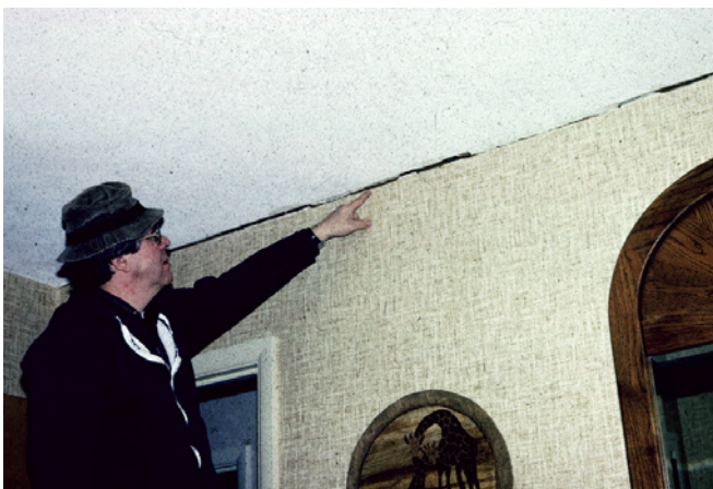
Photograph 4: Truss Uplift —Gypsum board ceiling cracks at interior wall ceiling connections due to truss uplift. Trusses move up in the winter and come down in the spring. Ah, the changing of the seasons, leaves change color and fall, and the trusses move up while the birds fly south.
