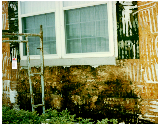
Photograph 3: Getting It Wrong – Water sensitive material in a highly insulated assembly with poor water management and a low drying potential. We needed a “pan flashing” under the window and a water control layer with a drainage gap over the OSB to control the wetting and no interior vapor barrier to permit inward drying. Can we say the 1800’s are calling with your safety factor....
