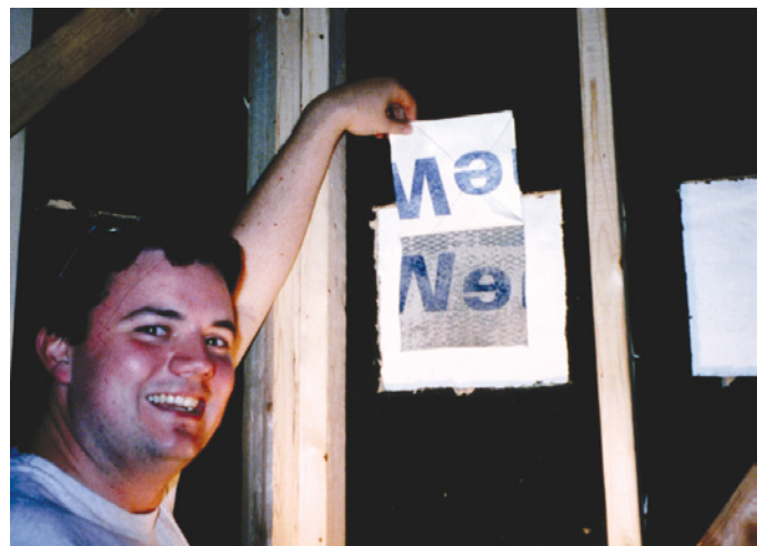
Photograph 6: Hardcoat Stucco Bonding to Plastic Building Paper —A young, happy engineer, discovers that stucco does indeed bond to plastic building papers preventing drainage. The engineer is my friend Chris Schumacher—may he remain this happy when he gets older.
