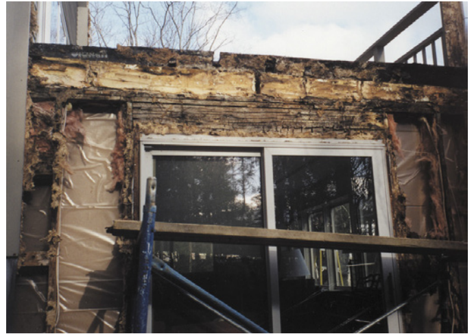
Photograph 5: Failure on Steroids —Note the plastic vapor barrier “accelerant” in this Vancouver, Canada building.
