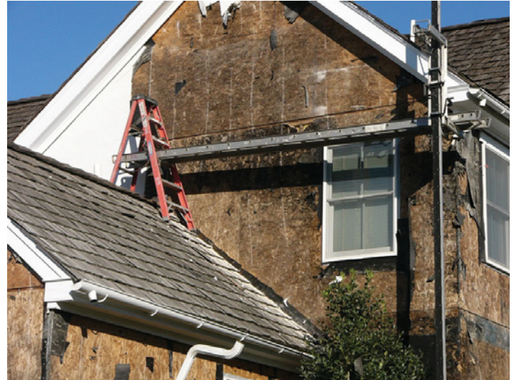
Photograph 4: Hardcoat Stucco Failures —Note that the damage is in the field of the wall away from windows.
