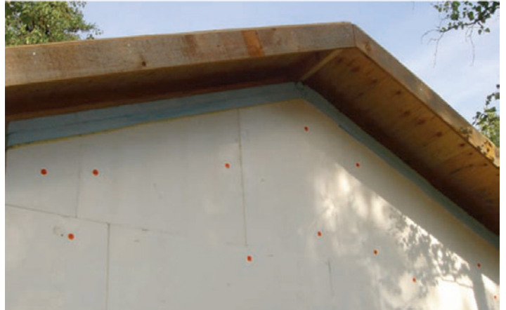
Photograph 4: Mock-up Constructed First —Things never go together perfectly the first time, which is why test huts, test sections, and mock-ups are essential. Again, ask me how I know. Failure is not an option north of the Arctic Circle. Skill testing question for the geeks in the audience: what are the red dots?
