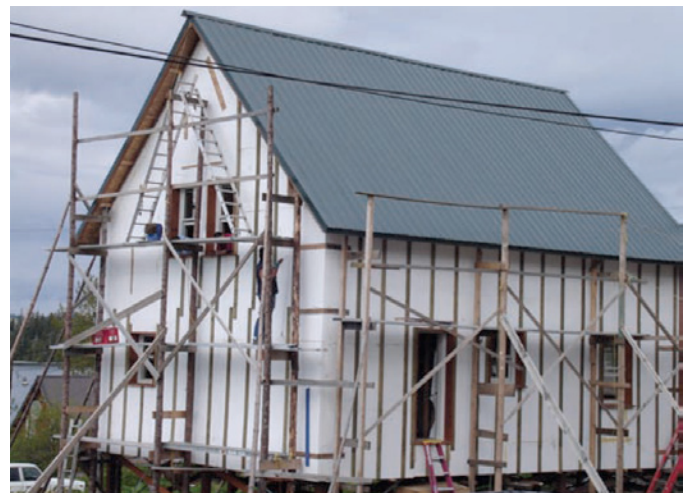
Photograph 2: Exterior insulation —Multiple layers of rigid insulation on the exterior of a wood-frame structure held in place with wood furring strips. Note the inset location of the windows allows the water management layer of the window to connect to the water management layer of the exterior wall (the fully adhered membrane).
