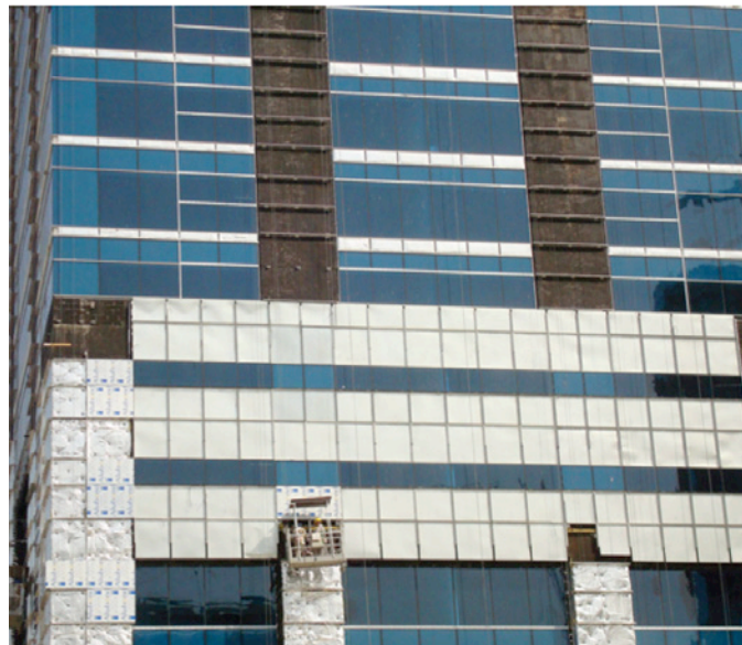
Photograph 7: Typical Dubai curtain Wall —The curtain wall is pretty much an uninsulated cladding that is installed over a CMU backup wall that is externally insulated with foil-faced rock wool. Note that the CMU is coated with a liquid-applied dampproofing. This is a good start. However, the liquid-applied dampproofings commonly used in Dubai are too thin to do much of anything. They don't do much for the rain control (but there is not much rain to worry about in Dubai). The key is that they are not effective air barriers as the assemblies are too air porous, and air barrier continuity is missing at punched openings (this is a big deal). This pretty useless thin stuff could easily be replaced with a "for-real" drainage plane/air barrier membrane (liquid applied) coupled with some minor detail changes at the punched openings. This change would be huge. Now, if you want to save costs, the CMU backup wall could be replaced with a steel stud wall with exterior paperless gypsum board. Think of the weight and resources saved? This configuration would actually be better than most curtain walls in Vegas, London, and New York. Oh, yeah, I almost forgot—the window area should be reduced, but you all knew that.
