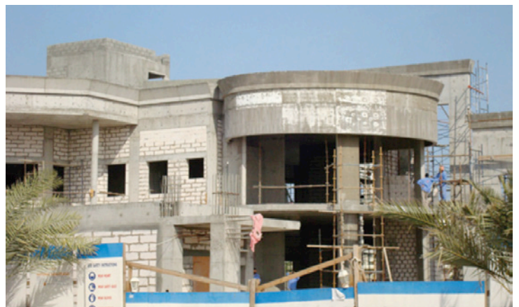
Photograph 4: Under the Dubai Stucco —Concrete masonry units are not insulated. Thermal resistance is nominally R-8. The roof membrane is installed over an unvented, uninsulated conditioned concrete slab. Thermal resistance is nominally R-8.
