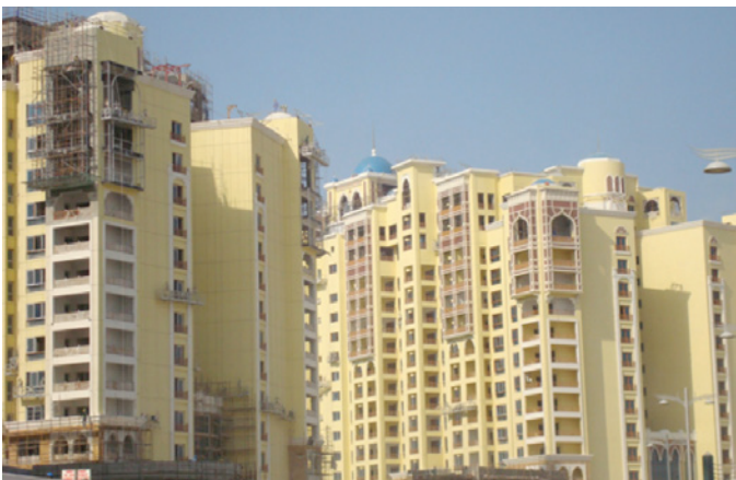
Photograph 6: More Dubai Stucco —Concrete frame, masonry backup wall has direct-applied exterior stucco. Thermal resistance is nominally R-8.
