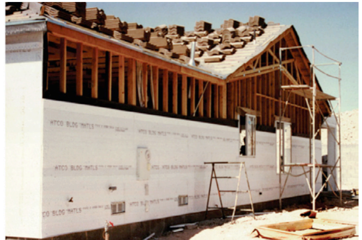
Photograph 3: Under the Las Vegas Stucco —Wood frame (2•6) externally insulated with expanded polystyrene installed over a drainage plane. Thermal resistance is nominally R-25. Tile roof is installed over unvented conditioned wood frame insulated assembly. Thermal resistance is nominally R-35.
