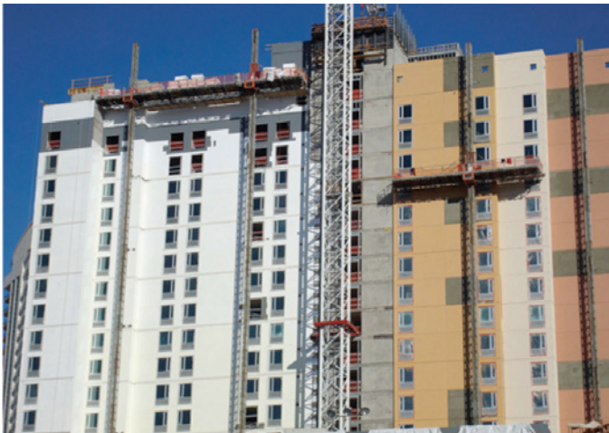
Photograph 5: More Las Vegas Stucco —Concrete frame, steel stud backup walls sheathed with paperless gypsum. Exterior insulation is EIFS. Thermal resistance is nominally R-20.
