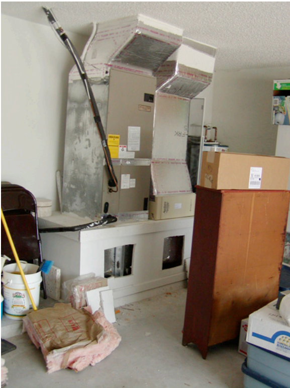
Photograph 6: Garage Return Platform —After a vented attic what is the worst possible place to locate an air-handler? Yes, you guessed it, the garage. Florida HVAC at its best.
