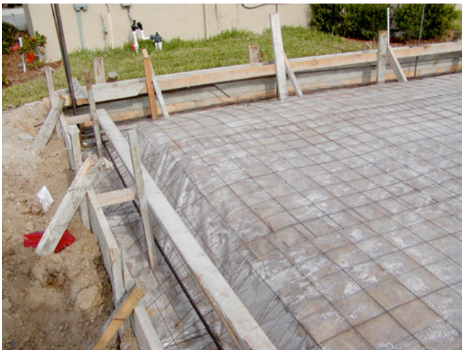
Photograph 2: Perimeter Capillary Break —Plastic sheet extends out under perimeter of slab edge foundation. Plastic skirt is attached to perimeter form boards protecting below grade portion of exterior slab edge.
