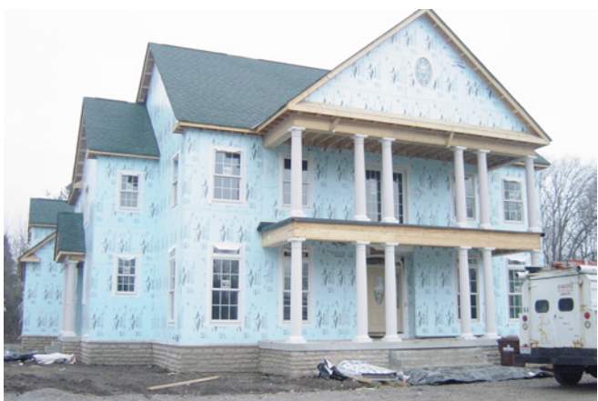
Photograph 2: Upstart? —Fifty years as a sheathing but still considered an upstart. Extruded polystyrene (XPS) completely sheathing the structure – continuous thermal break. “Beginning show up on the range...confusing the cowboy builder and architect...”
