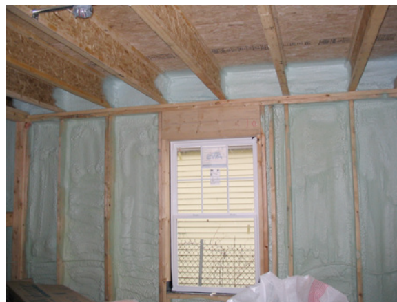
Photograph 5: High-Density Spray Foam Cavity Insulation —High tech and low perm. Great air sealing, great thermal performance, great structural strength. Does not allow for any appreciable inward drying of the exterior sheathing.
