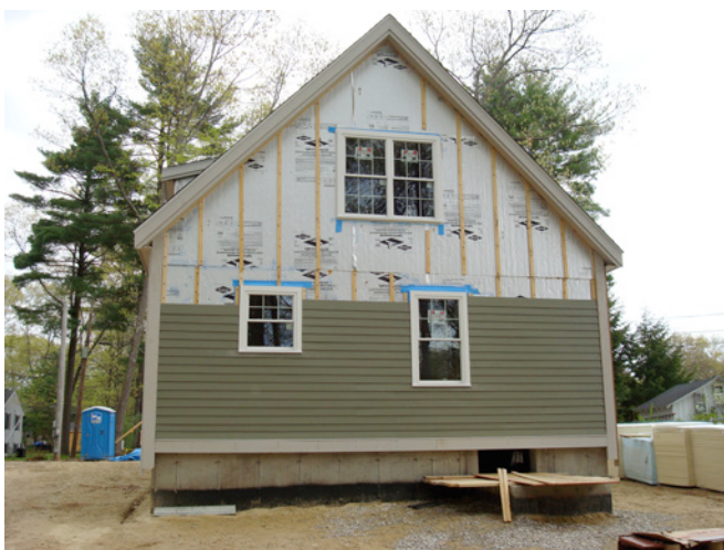
Photograph 7: Furring —When foam sheathings exceed 2 inches in thickness 1x4 furring becomes necessary. This wall has 4 inches of foil-faced polyisocyanurate insulating sheathing installed over a 2x6 wood frame wall. The wood furring acts as the nail base for the fiber-cement cladding.
