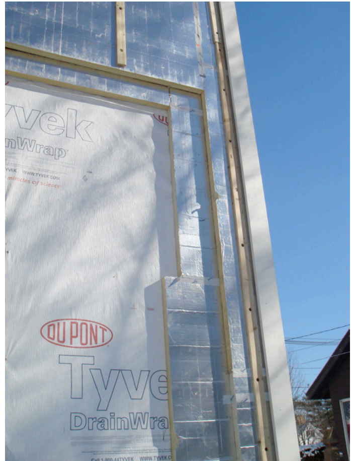
Photograph 11: Perfect Wall Redux —The almost perfect wall has “crinkled” housewrap providing hygric redistribution, 4 inches of foil-faced polyisocyanurate insulating sheathing providing the ultimate thermal break, wood furring providing cladding attachment, relief of hydrostatic pressure and back-ventilation of cladding. OSB under the housewrap provides shear and high-density spray foam cavity insulation (obviously hidden from view) provides air sealing and even more thermal performance. Who says that all these products can’t get along?
