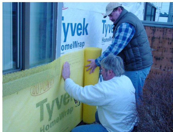
Photograph 3: “High-tech air?” —Polypropylene mesh providing an air gap between OSB covered with housewrap and cladding.
