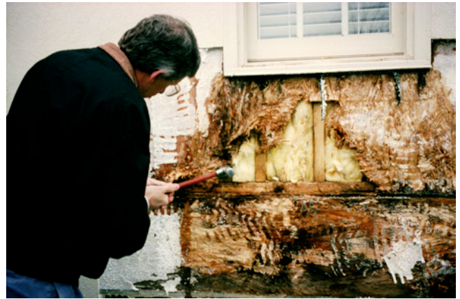
Photograph 8: Nightmare —Exterior Insulated Finish System (EIFS) directly adhered to water sensitive OSB sheathing. Water passes through and around stucco cladding and is trapped between the foam sheathing and the OSB. Water-managed EIFS does not have this problem and is an awesome system.
