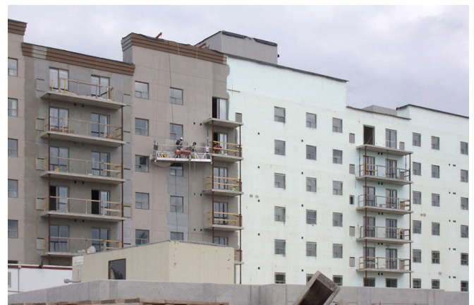
Photograph 2: Thermally Broken Balconies —Clip on balconies where exterior balcony corners are supported by columns supported by the balcony below.
