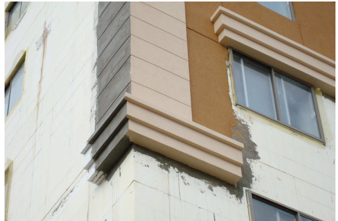
Photograph 4: Synthetic Stucco Rendering —Complex aesthetics are possible and typical.
