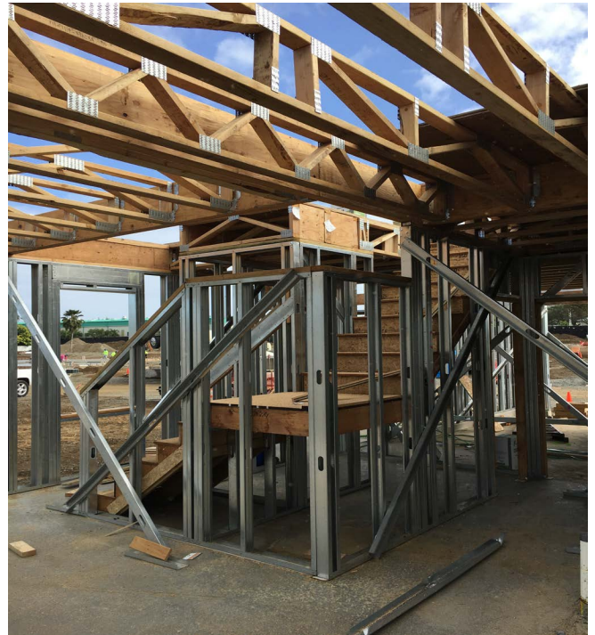
Photograph 6 – Minimize Wood: It is impractical to get rid of all wood. So you minimize it and move it up away from the ground and those miserable termites.
