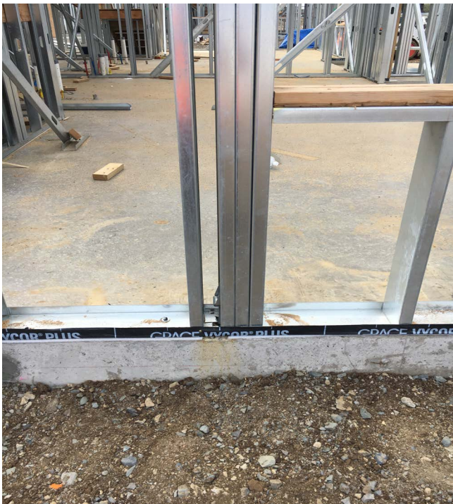
Photograph 5 – Steel Rusts: Termites don't eat steel. Not a lot of wood stud framing. But steel rusts. Where the steel framing is in contact with the concrete slab the bottom track of steel is wrapped with a peel and stick membrane to reduce the risk of corrosion.
