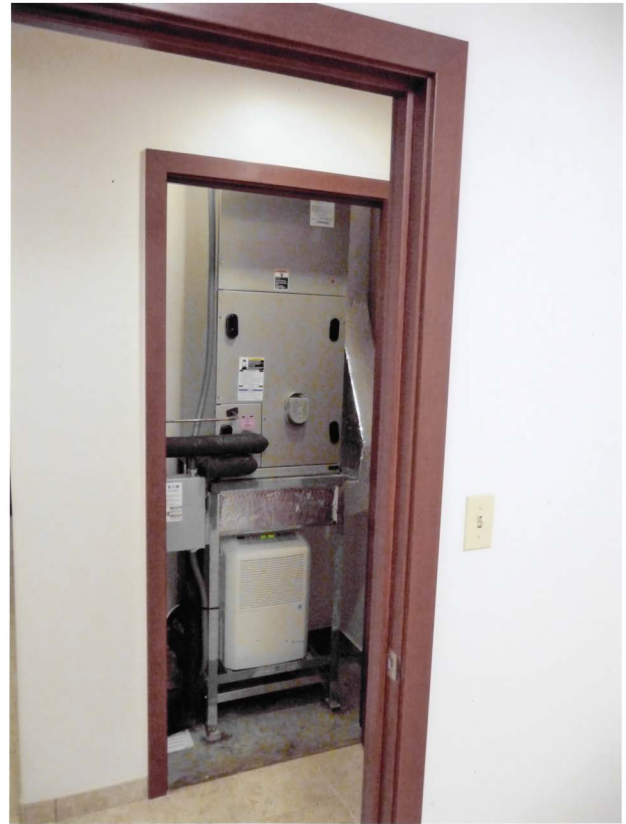
Photograph 11 – Dehumidifier: Still have a part load humidity problem to deal with. We have great windows, lots of thermal insulation, compact fluorescent and LED lights, and controlled ventilation. Not much of a sensible load. We do have a big latent load. We have to remove the humidity. Yup, we need a dehumidifier.
