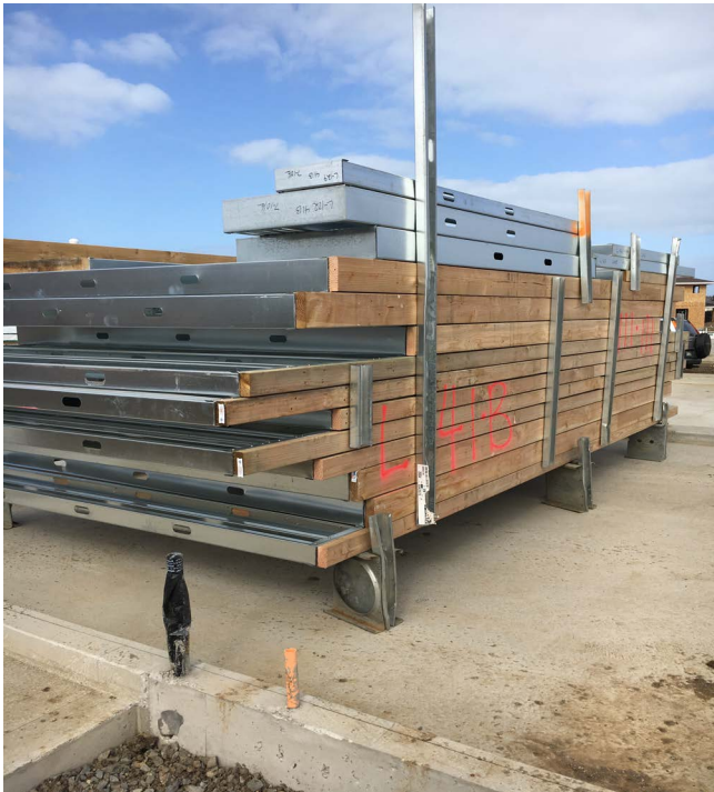
Photograph 4 – Steel Framing: Even with steel framing we typically have a wood top plate and wood framing around punched openings such as windows.
