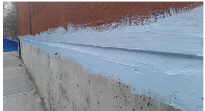
Photograph 8 – Continuous Seal: Note the “airtight” seal between the sheathing and the concrete foundation. We do not want “salty” air getting into the wall framing and causing havoc with our steel studs and connections.
