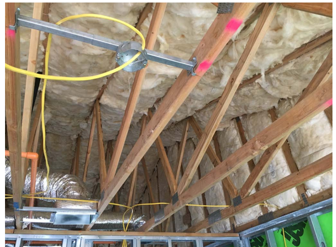
Photograph 9 – Hawaiian Roofs: Don’t vent roofs in Hawaii. Move the insulation from the “flat” to the “slope” and install a vapor diffusion ridge vent to allow vapor to exit the assembly via vapor diffusion. No air change between the attic and the exterior occurs. This has three huge benefits. First, no salty air into the attic and no corrosion. Second no exterior humid air into the attic to cause ducts to sweat and a huge increase in airtightness of the entire assembly reducing part load humidity problems and providing a huge thermal benefit. Third, the ducts are now in conditioned space providing a huge thermal benefit.
