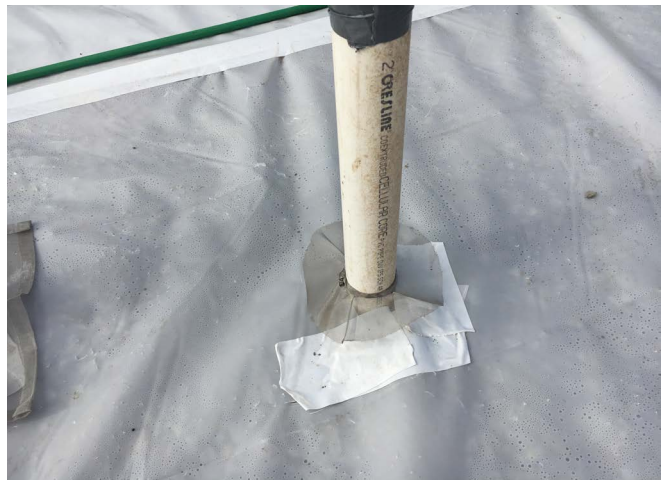
Photograph 3 – Physical Barrier: Even better, note the stainless steel mesh clamped to the pipe penetration that gets cast into the slab creating a physical termite barrier.
