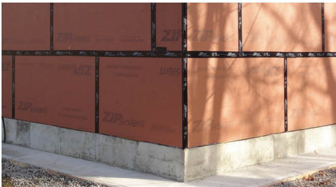
Photograph 7 – OSB Sheathing: Note the integral water control layer on the face of the OSB. The joints in the OSB are taped to provide water control layer continuity and air control layer continuity. The OSB also acts as a “vapor throttle” reducing inward vapor drive. Note in hot, humid climates the dominant vapor flow is from the outside to the inside. Also note the “concrete skirt” around the perimeter of the foundation to keep insects, vermin and plant growth away from “where the building touches the ground”. More “physical barrier” stuff. Don’t knock it, it works.
