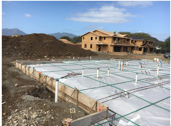
Photograph 2 – Slab Done Right: Note the complete polyethylene ground cover, taped joints, wrapped under the perimeter slab edge and tied into the perimeter slab forms with a polyethylene “hem”. The ground is treated under the slab and at the slab perimeter with fipronil prior to the installation of the polyethylene ground cover.
