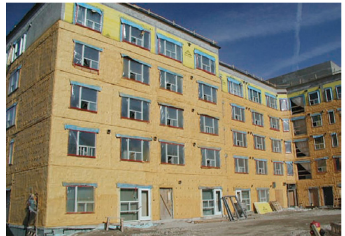
Photograph 1: The Perfect Wall?
