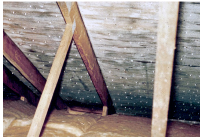
Photograph 3: Roof Sheathing —Nails frost up first, then the underside of the roof sheathing.
