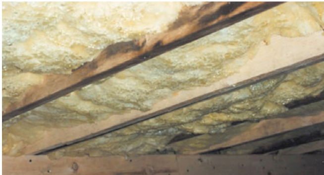
Photograph 5: Crawlspace Condensation —Water droplet forest on underside of crawlspace subfloor cavity insulation.
