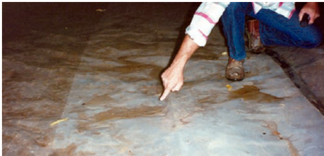
Photograph 6: More Crawlspace Condensation —How did the water get on the top of the plastic ground cover? It condensed out of the ventilation air.
