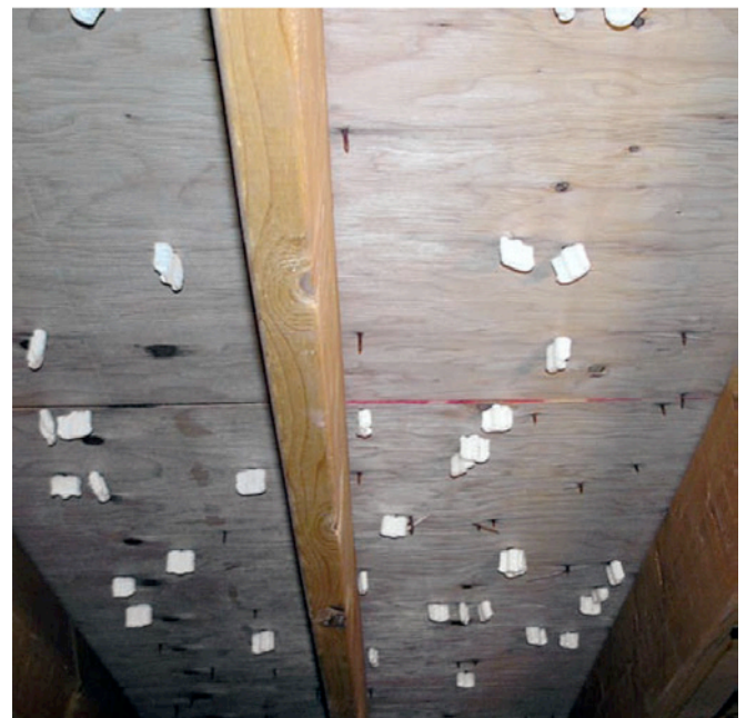
Photograph 4: Condensation Control —Yes, it is true, there are crazy people around. An attempt to warm nails by insulating them.
