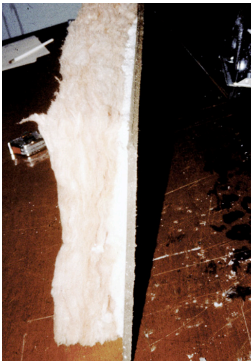
Photograph 1: Surfaces are Where the Action Is —The frost has accumulated at the backside of the sheathing, not in the middle of the cavity insulation.
