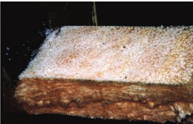
Photograph 7: Radiation Coupling in Attic —Frost on the top surface of attic ceiling insulation.
