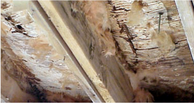
Photograph 10: Condensation and Decay are Bad —Air permeable insulation under deck can lead to condensation and decay. You would never construct an unvented roof this way. So why would you ever construct a deck this way?
