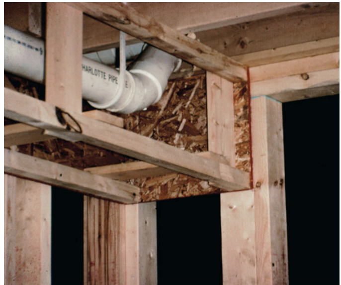
Photograph 9: Draftstopped Soffit —'Nuff said.
