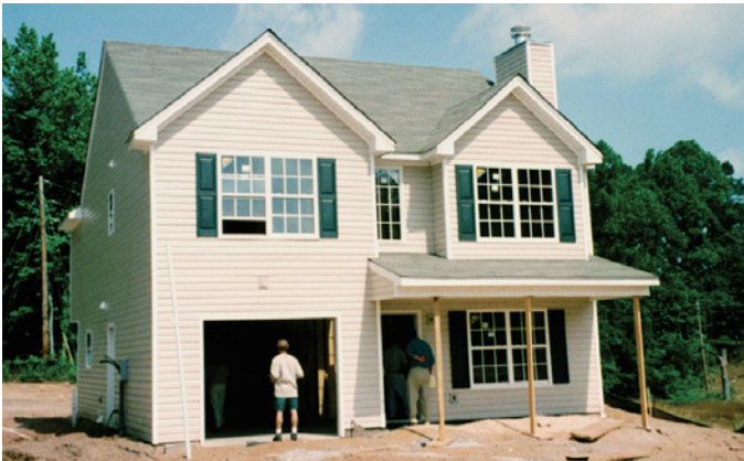
Photograph 10: Bedroom Over Garage —Unfortunately, in my experience, garages are not effectively isolated from houses, especially at the second floor assembly to interior garage perimeter.
