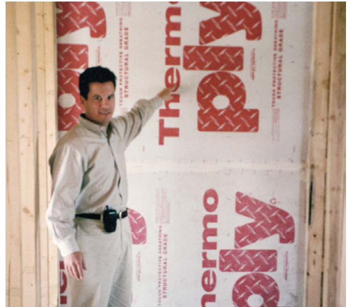
Photograph 6: Tub on Exterior Wall Before Tub Installation —Notice the rigid material on the exterior wall where the one-piece shower/tub thingy is going to be.
