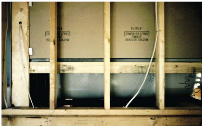
Photograph 2: Bathtub on Exterior Wall —The classic “Joe Hole”—a hole so big even I can crawl through it. It needs to be draftstopped with something rigid and airtight. Note to folks out there in the real world: fluffy insulation is not rigid and airtight. But a sheet of OSB or gypsum board over fluffy insulation makes the fluffy insulation happy and Joe happy.
