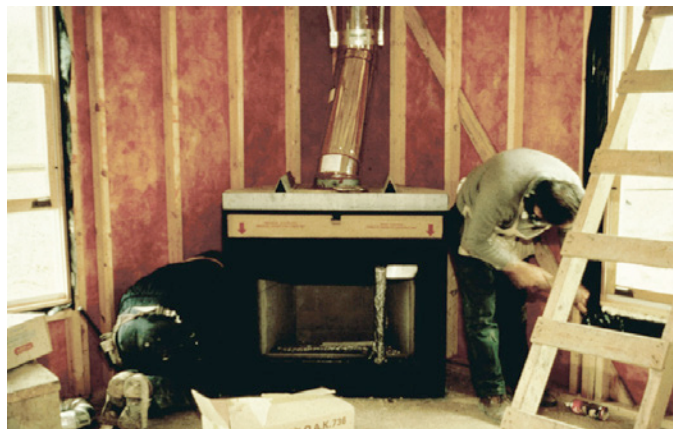
Photograph 3: Fireplace on Exterior Wall —OK, an even bigger hole than the bathtub hole. Kind of makes it funny to think about sealing an electrical wire going through a top plate when you have something this big.
