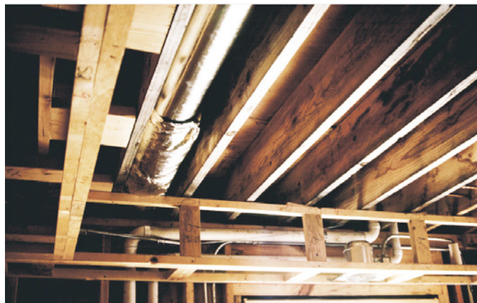
Photograph 4: Soffit on Exterior Wall —Wow, this allows for connecting your entire floor cavity to the outside.
