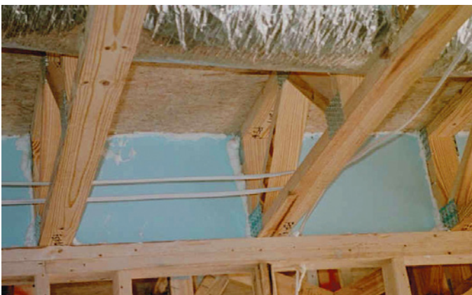
Photograph 11: Bedroom Over Garage Done Well —Notice how beautifully the floor joists are draftstopped over the top of the wall that separates the interior garage perimeter from the house. This location typically represents a huge leakage area (aka, big holes).
