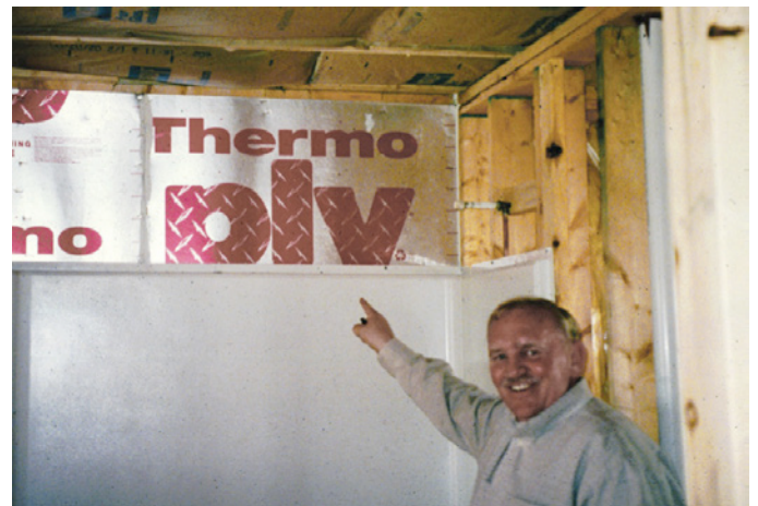
Photograph 7: Tub on Exterior Wall After Tub Installation —Notice the rigid material on the exterior wall behind where the one-piece shower/tub thingy is. Notice the even bigger smile on that VP of construction.
