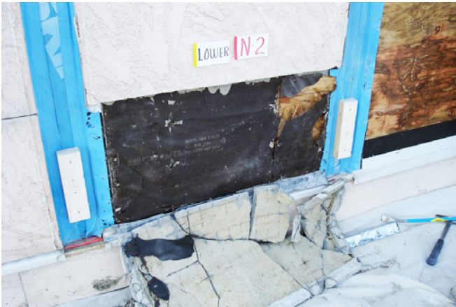
Photograph 6: Stucco over OSB Wall - North elevation deconstruction of hard-coat stucco applied over building paper over OSB.
