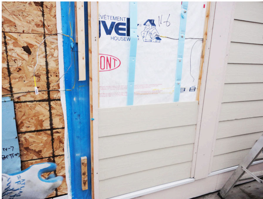
Photograph 10: Fiber cement siding - If you install a polyethylene vapor barrier on the inside of your wall and you sheath it with OSB you had better back ventilate your external cladding. It makes a big difference. Note the “blue” spacer strips that create a \frac{3}{8} -inch ventilation and drainage gap between the siding and the water control layer.
