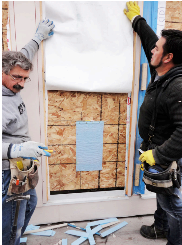
Photograph 9: Exterior Wetting Apparatus – Note that the capillary active mat used to distribute water injected behind cladding is located behind the water control layer directly over the exterior surface of the OSB sheathing.
