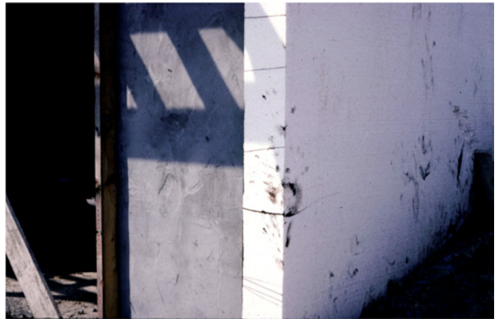
Photograph 2: Air Control Layer – Cement rendering is the air control layer. Mechanically attached 8 inch thick expanded polystyrene (EPS).
