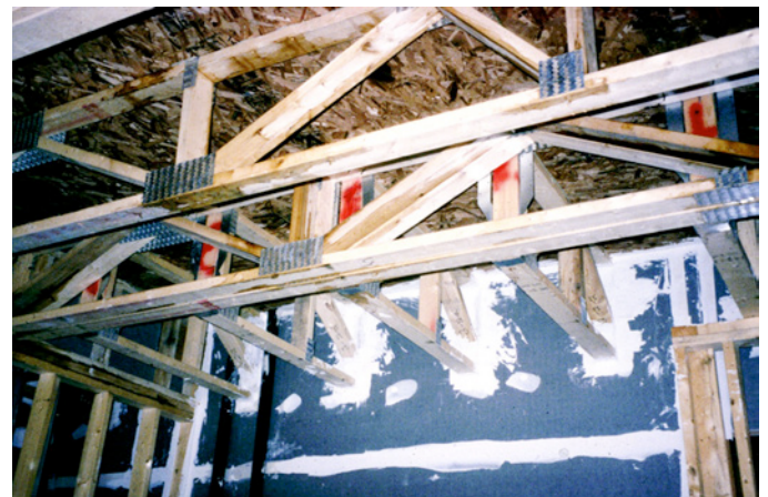
Photograph 1: Compartmentalization Air Sealing —Gypsum board is run up to the underside of the floor sheathing above and sealed with joint compound.
