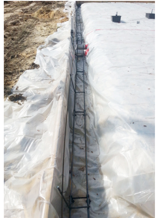
Photograph 2: Perimeter Slab Protection —The plastic vapor barrier is run over the top of the form boards and trimmed later after the form boards are stripped.
