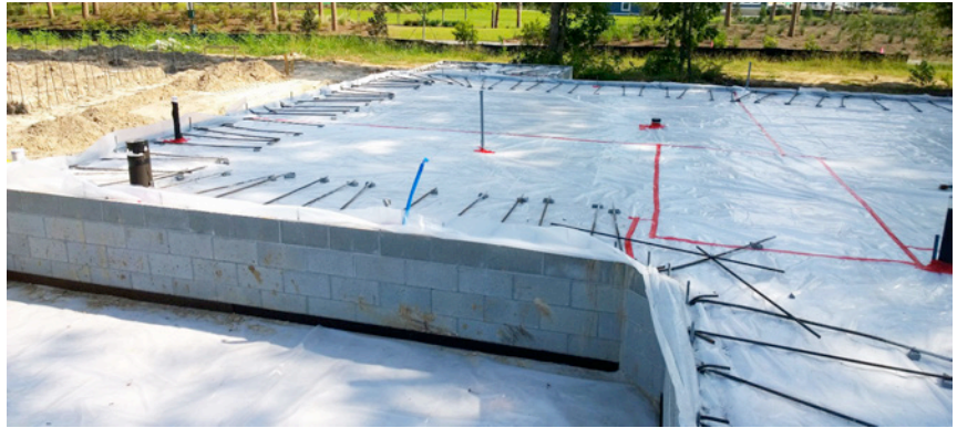
Photograph 4: Stem Wall Foundation —It is a lot easier to handle a stem wall foundation where the edge of the slab is wrapped and the slab is well elevated.
