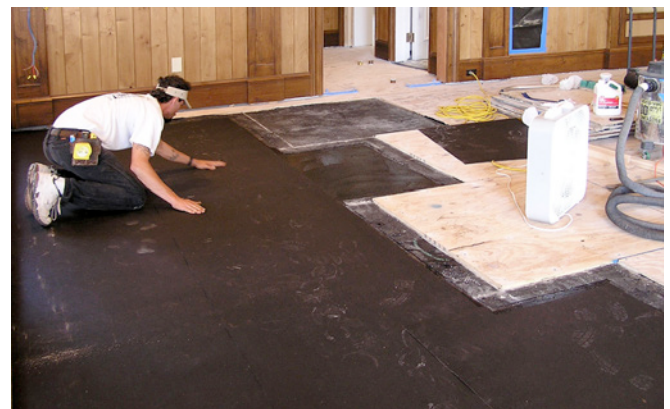
Photograph 1: Plywood Over Bitumen —Plywood replaced wood sleepers and was covered with a slip surface to keep the wood flooring from squeaking as it changed moisture content seasonally.
