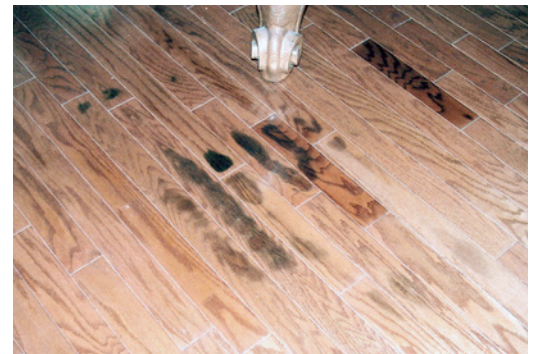
Photograph 3: Wood Flooring Problems —Discoloration, movement and decay.
