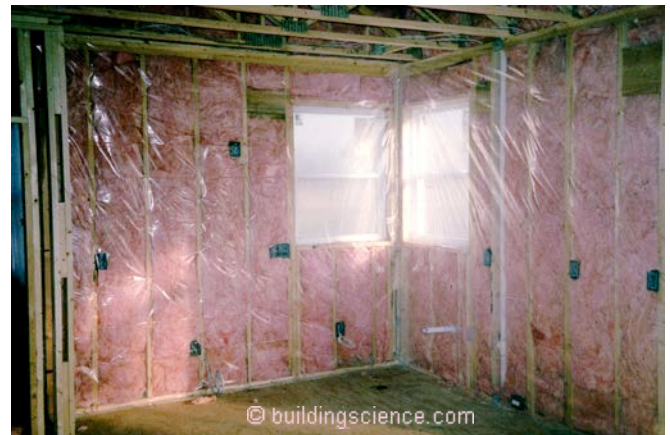
Photograph 1: Plastic Vapor Barrier —Not a “production friendly” method of achieving airtightness and it was not “robust” in terms of surviving the construction process and in providing performance over the service life of the building. It was also climate sensitive. It made no sense for assemblies that saw air conditioning – it was a vapor barrier on the wrong side of such assemblies.
