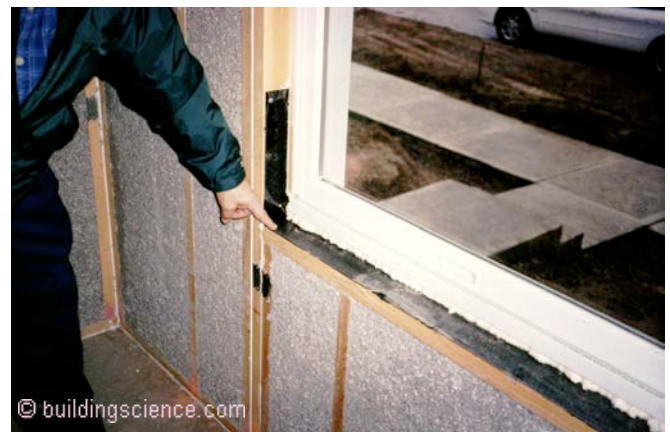
Photograph 2: Interior Gypsum Board as the Air Barrier —Note the sealant at the bottom plates an around window openings.
