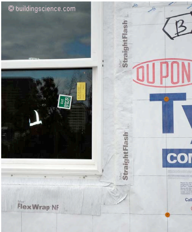
Photograph 7: Robust Rainwater Control —Numerous elegant and clever accessories were introduced to deal with rainwater control particularly at window-to-wall interfaces. This is a formable and flexible membrane “pan flashing” system.
