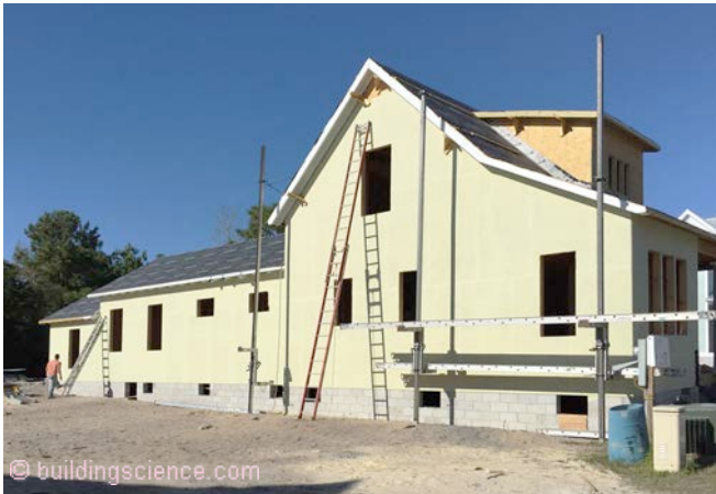
Photograph 11: Water Control/Air Control Continuity —The fluid applied coating must connect to the air control layer of the roof assembly and to the air control layer of the foundation assembly.
