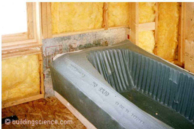
Photograph 3: Bathtub on Exterior Wall —Targeting the big holes with rigid draft-stopping. Of course an even better approach is not have a bathtub on an exterior wall...
