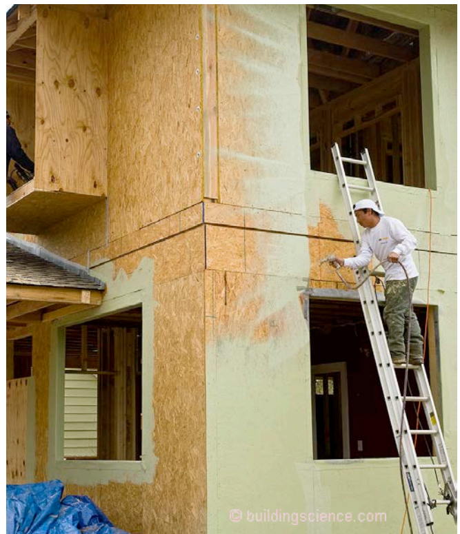
Photograph 10: Fluid Applied Air Barrier —The coatings needed to be able to span joints and they needed to be vapor permeable. And their most important function, rainwater control could not be compromised.
