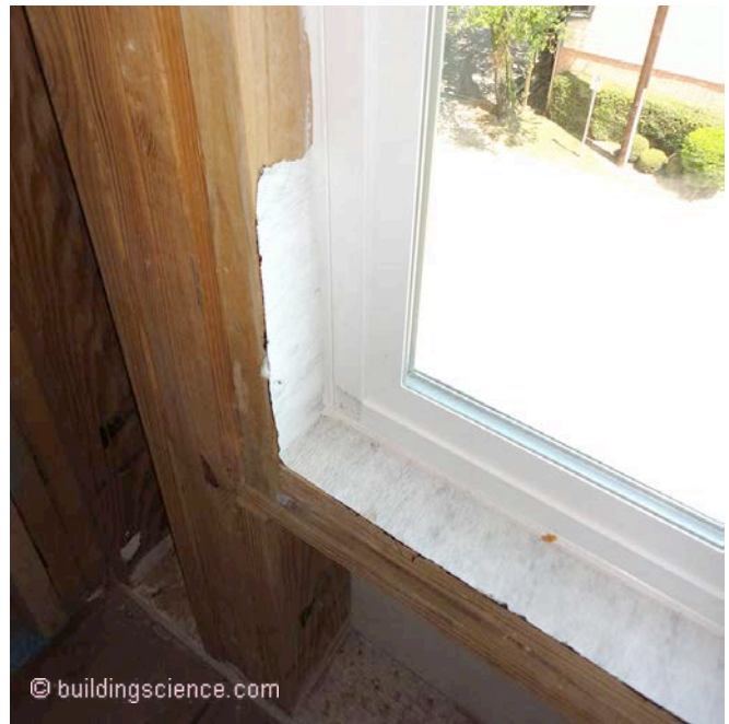
Photograph 8: More Robust Rainwater Control —Beautiful “under window gutter” where the pan flashing is sealed to the interior of the window unit for air barrier continuity.
