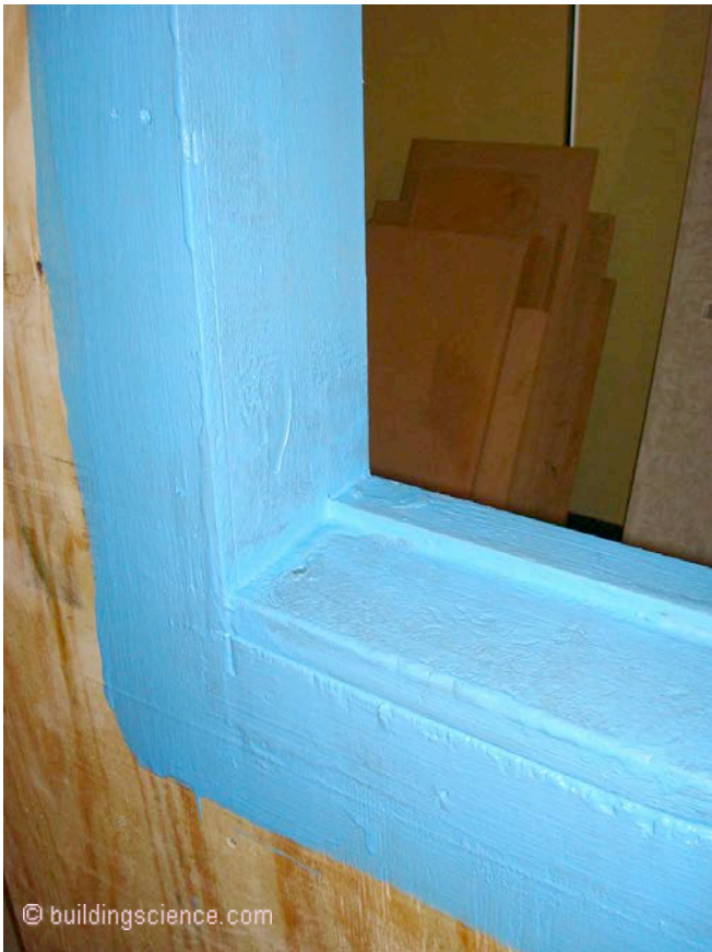
Photograph 12: Window Opening —Origami is not a necessary skill with fluid applied flashing systems.
