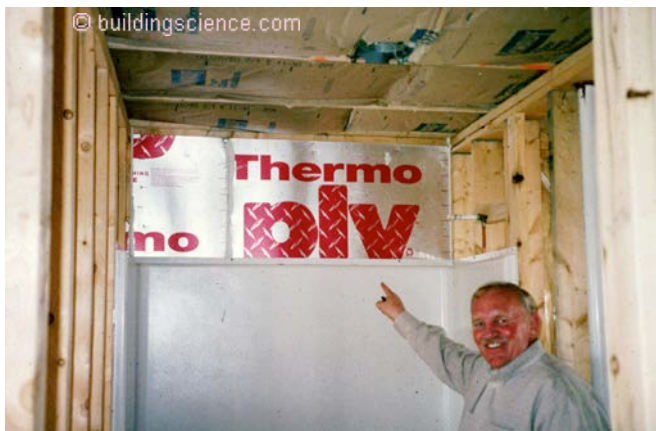
Photograph 4: One-Piece Tub Shower Enclosures —A really, really big hole on an exterior wall sealed by a very happy builder. Note the sealant around the perimeter of the rigid draft-stopping sealing the draft-stopping to the framing.
