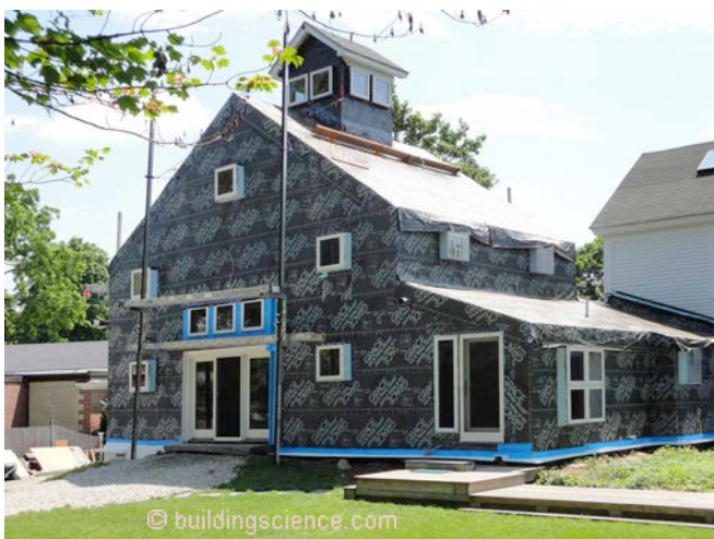
Photograph 9: Fully Adhered Membrane —Ultra high levels of airtightness with ultra high levels of cost. Not the easiest stuff to install either. I should know, this is my place.
