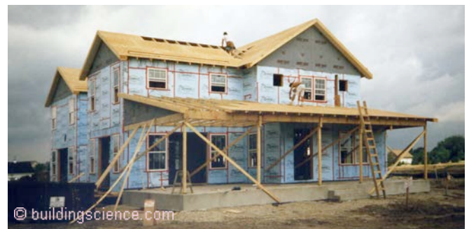
Photograph 15: Insulating Sheathing Water and Air Control Layer —The insulating sheathing provides three functions in this approach – water control, air control and thermal control.
