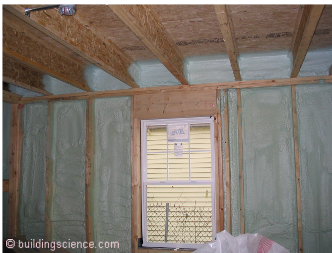
Photograph 5: Interior Spray Polyurethane Foam —In frame construction, spray foam is not continuous at all wood-to-wood connections. These details need to be addressed.
