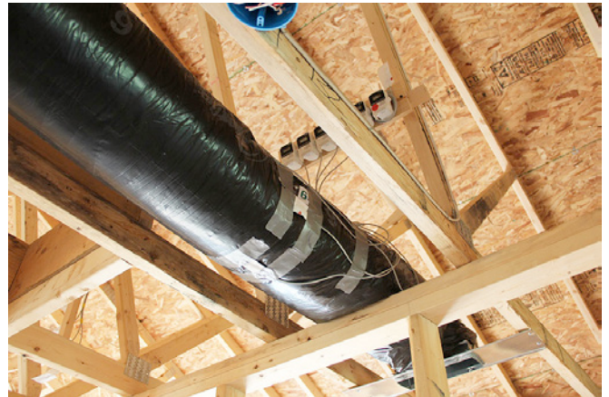
Photograph 8: Test House Instrumented Ductwork - Ductwork surface condition instrumentation.
