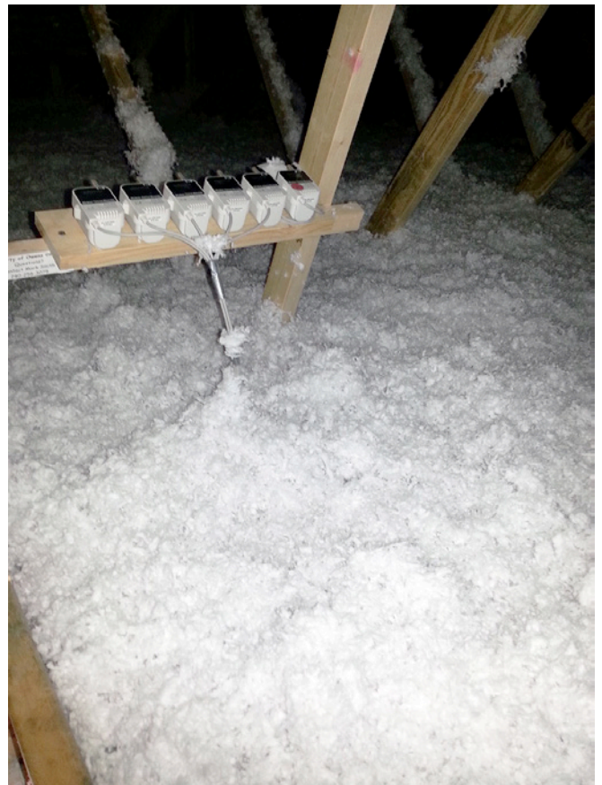
Photograph 9: Test House Attic – Loose fill insulation burying instrumented ductwork.
