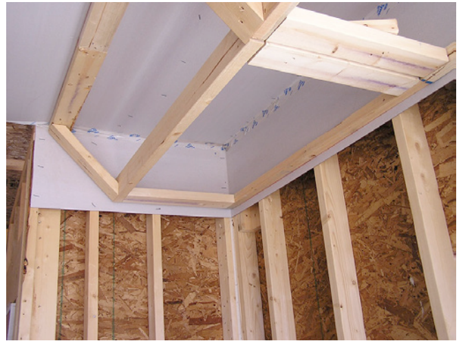
Photograph 1: Dropped Ceiling Framing - It is not easy to go to dropped ceilings. It is expensive* and it is difficult to make the ceiling plane “airtight” above the dropped ceilings.
