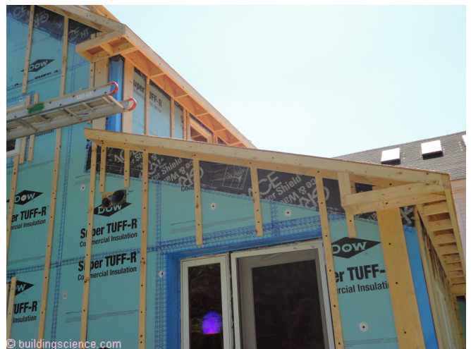
Photograph 4: Robust Connections - Roof eaves and roof rakes experience the highest positive and negative air pressures. The structural connections connecting the roof deck layers to the wall assemblies need to be “robust”.
