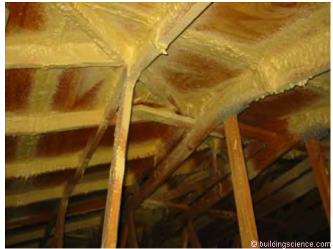
Photograph 3: Retrofit Repair – In retrofit applications it may be possible to seal the sheathing joints from underneath using closed cell, high density spray polyurethane foam (SPF). Photograph courtesy of The Insurance Institute for Business & Home Safety (IBHS).
