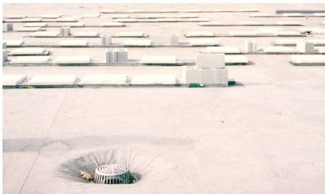
Photograph 2: Membrane Flutter Repair – Yes, this is done more often than we would all like to admit.
