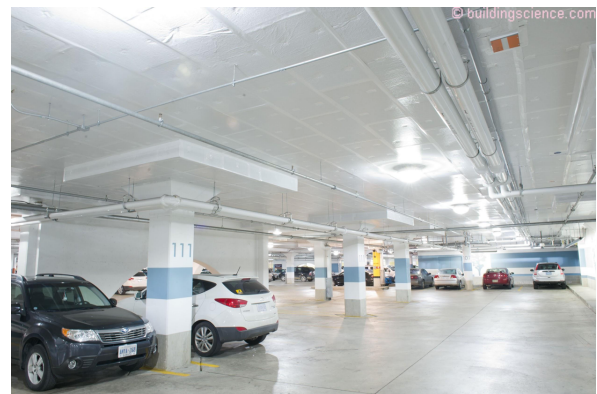
Photograph 1: Faced Fiberglass or Mineral Wool Insulation – The insulation is mechanically attached to the underside of the structural slab and joints and seams taped.
