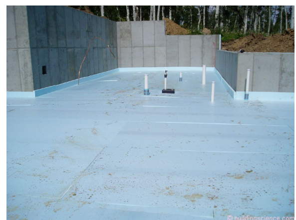
Photograph 2: Floor Slab Insulation - Continuous rigid insulation is located under the basement floor slab. This insulation can be any rigid insulation product. All work is installed over a granular layer.
