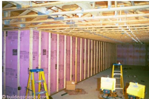
Photograph 3: Frame Wall – An insulated frame wall assembly can be located to the interior of the interior rigid insulation.
