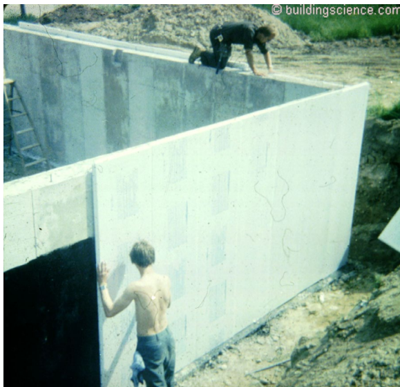
Photograph 4: Exterior Rigid Insulation – Extruded polystyrene is installed on the exterior of the concrete foundation wall.
