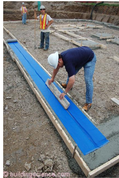
Photograph 1: Dampproofing Footing – Dampproofing the top of footings controls capillarity at this location. Footing dampproofing can be fluid applied or a fully adhered membrane
