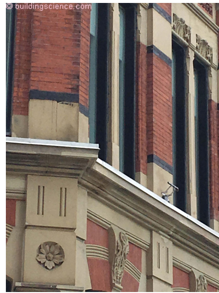
Photograph 10: Montreal Retrofits - Look at the retrofitted drip edges that are going hand-in-hand with the energy efficient window replacement and interior insulation.
