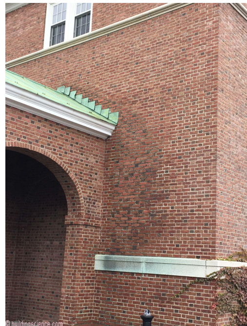
Photograph 14: Bad Detail - Dumping the roof rainwater runoff right on the wall is a bad idea.
