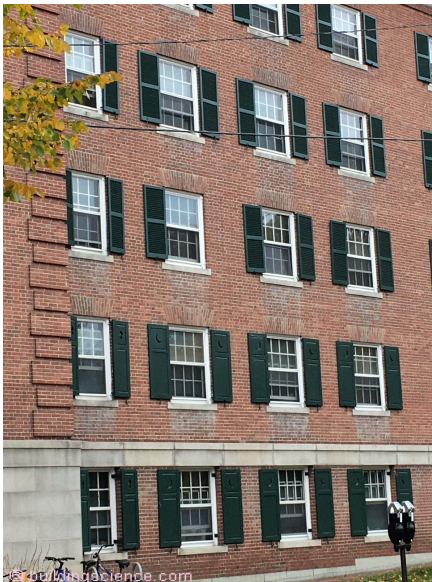
Photograph 3: Surface Tension Rainwater Stains - no kerf...no drip...
