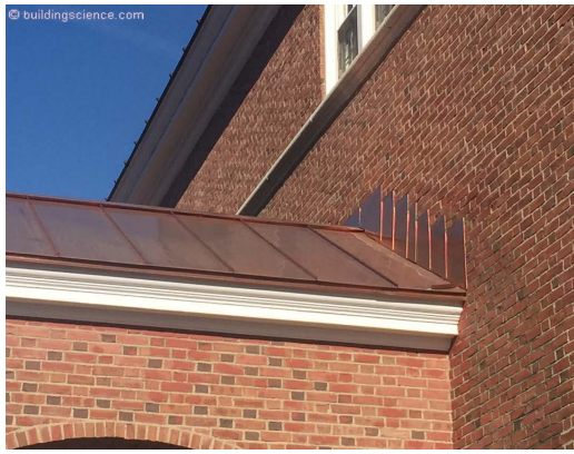
Photograph 15: Bad Detail Repaired - Elegant fix that is pretty much invisible. A “minor” “kick out” with a “major” impact...a short diagonal metal roofing “ridge” directing water away from the roof/wall interface.
