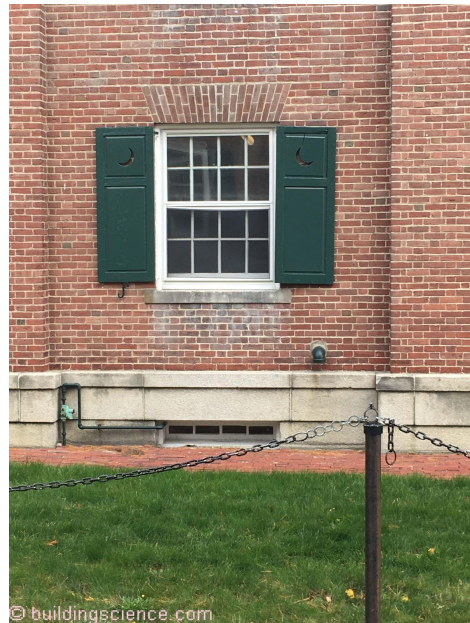
Photograph 4: Surface Tension Rainwater Stains - no kerf...no drip...
