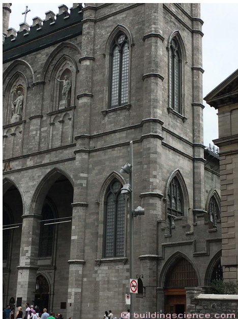
Photograph 7: Notre-Dame Basilica in Montreal – Deuxième partie – Original “drip edges” did not work...they got retrofitted with lead coated copper drips.
