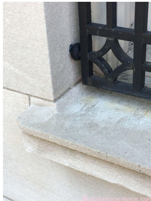
Photograph 1: Stone Sill - Beautiful sloping stone sill...sloping from the back...and from the ends...and look at the front edge drip.
