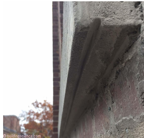
Photograph 5: Retrofitted Kerf – A kerf can easily be retrofitted with a Skilsaw and a diamond blade. Even better, the kerf is invisible.
