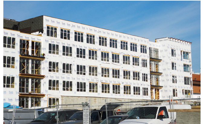
Photograph 3: Multifamily —Sheet vapor permeable water control layer and air control layer. The “classic” air infiltration barrier that also controls rainwater installed on the exterior of vapor permeable sheathing such as glass faced gypsum board.
