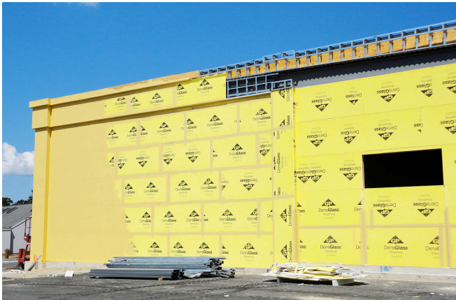
Photograph 2: Commercial/Retail —Fluid applied vapor permeable water control layer and air control layer installed over a vapor permeable glass faced gypsum board.
