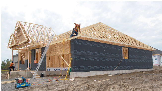
Photograph 1: Residential —Fully adhered vapor permeable water control layer and air control layer. Yes, one material or product can do both things. Note the now typical oriented strand board (OSB) sheathing—a semi-vapor permeable material—an “external vapor throttle”.
