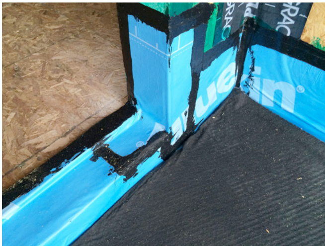
Photograph 5: Drainage Matt —Membrane waterproofing is stripped into the pan flashed balcony door opening. Note the drainage mat installed over the top of the membrane waterproofing. Also note the mastic application sealing the vertical portion of the balcony deck waterproofing membrane to the wall sheathing.
