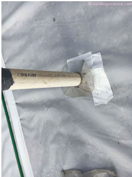
Photograph 6: Plumbing and other services that penetrate concrete slabs are sealed with a stainless steel mesh “skirt” clamped to the service penetration. The mesh is subsequently cast into the concrete.
