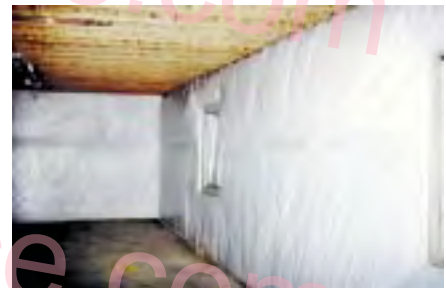
Photograph 3 Blanket insulation with impermeable vinyl interior surface
