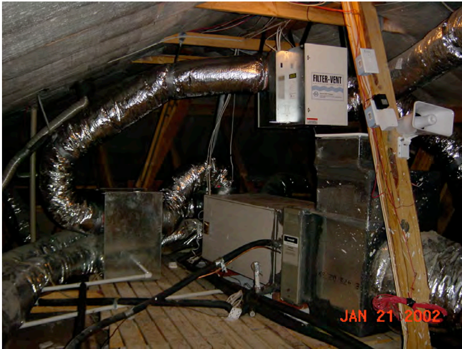
Figure A-4a Photograph of Filter-Vent system with ducted dehumidifier in conditioned attic
