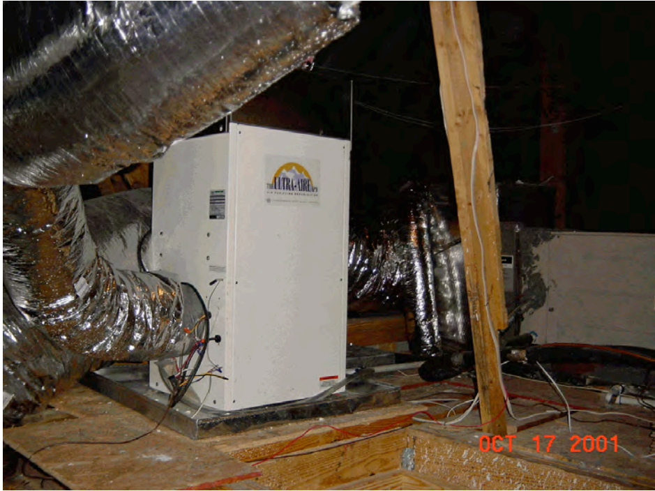
Figure A-3a Photograph of UltraAire system located in conditioned attic
