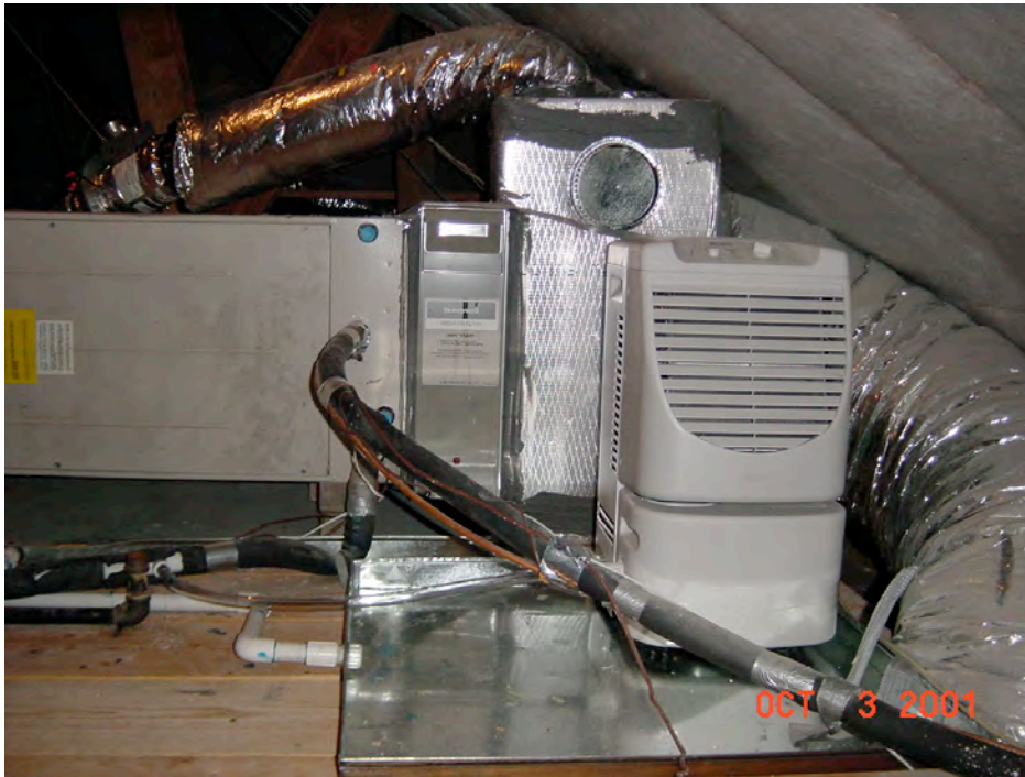
Figure A-2a Stand-alone dehumidifier in conditioned attic
