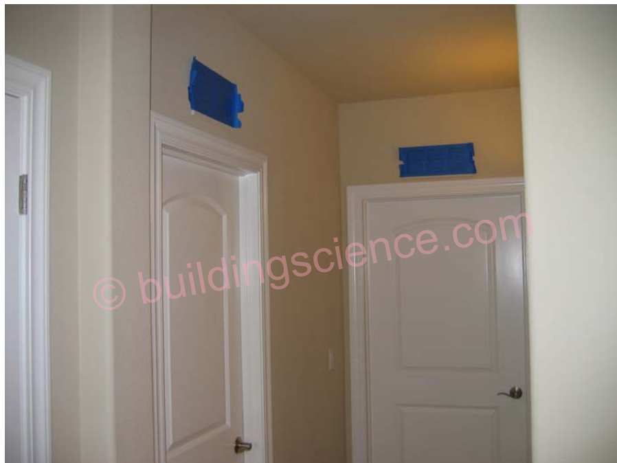
Figure 24. Transfer grilles over bedroom doors taped closed.
