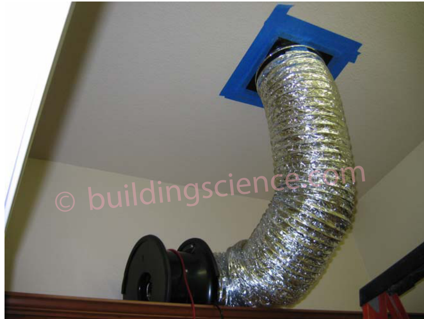
Figure 7. Duct Blaster® installed at the laundry room exhaust register.
