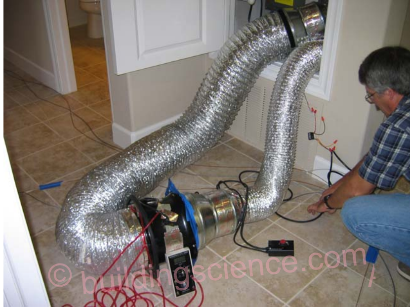
..... Figure 8. Duct'Blaster installed between the outside air duct ..... and the return of the air handler to provide supply ventilation.
