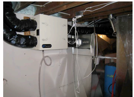
■ Heat recovery ventilator (HRV) installed in a basement, connected to a central air handler system
