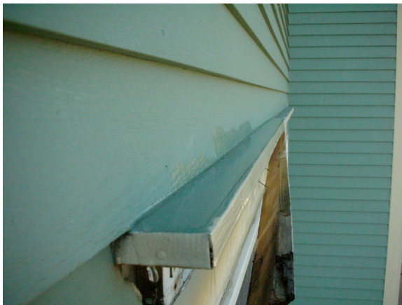
Improper sloped head flashing directing water back towards the building
