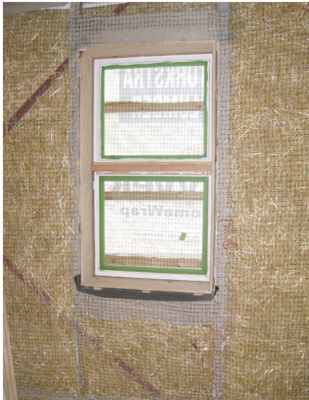
Photograph 3: Window framing (with subsill flashing), shear bracing and wire mesh reinforcement. This wall is ready for plaster.
