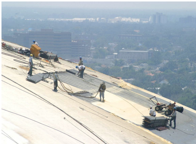
Photograph 5: Spray Foam Application —New, fully adhered roof insulation and integral air barrier.
