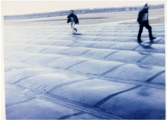
Photograph 2: Fluttering Membrane —No air barrier at deck leads to an idea for a Disney World ride...
