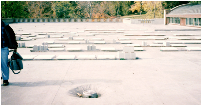
Photograph 3: Fluttering Membrane Fix —“I’ll fix that darn moving membrane, Bubba get me some pavers and blocks...”
