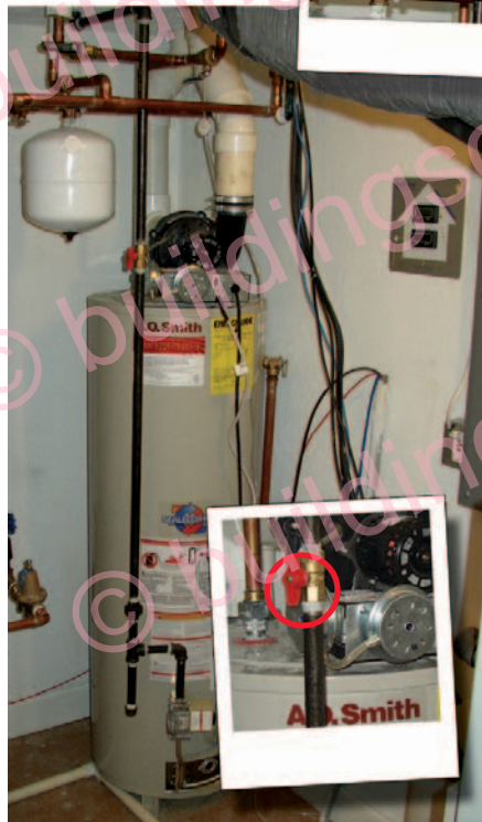
Hot water heater with main water shut-off (inset top) and gas shut-off to unit (inset bottom). Note the SunChoice™ control panel on the wall to the right of the water heater.
