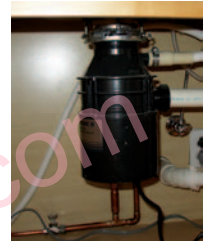
Garbage disposal located under kitchen sink
