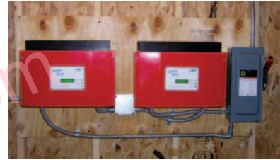
The inverters are located in the garage
