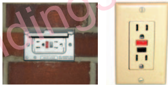
GFCI outlet inside (right) and outside (left)
