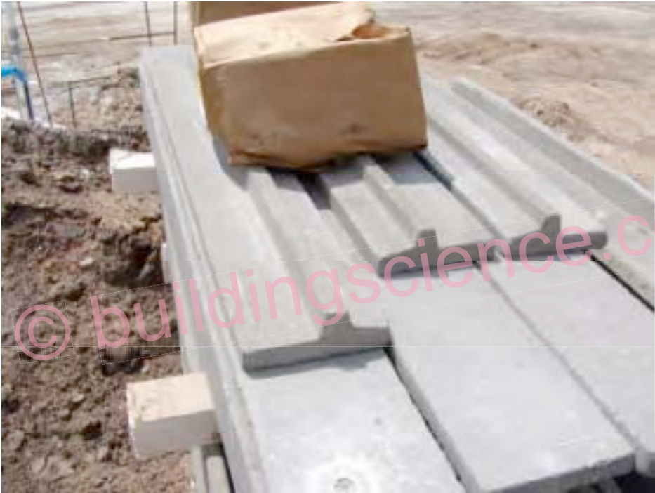
Photograph 27: Precast Sill With Illogical Attachment Rib
