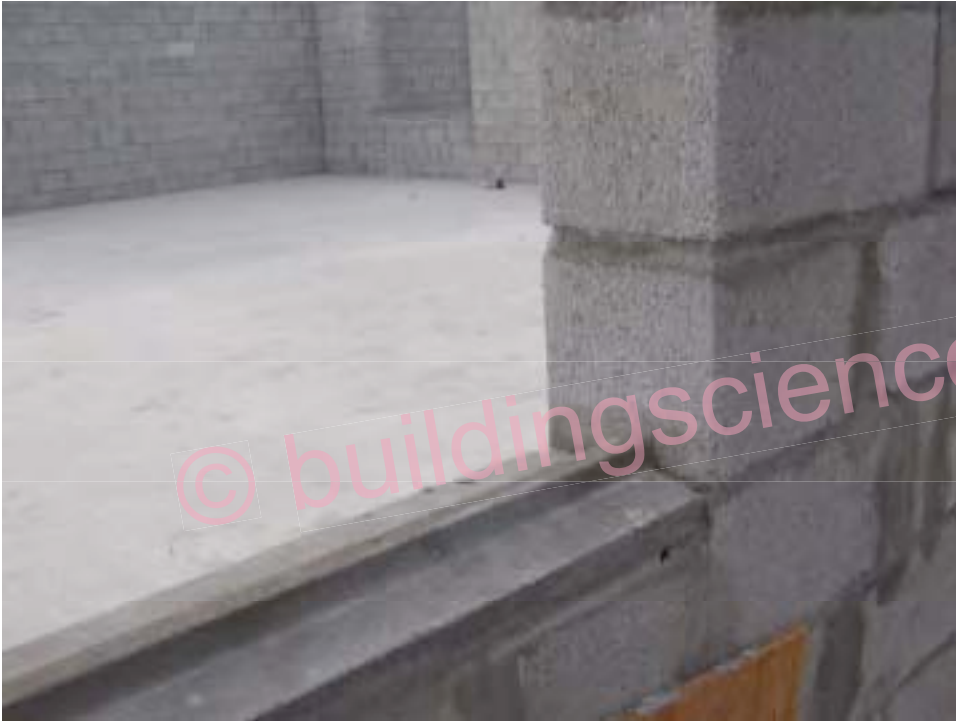
Photograph 28: Precast Sill That Channels Window Leakage Inward
