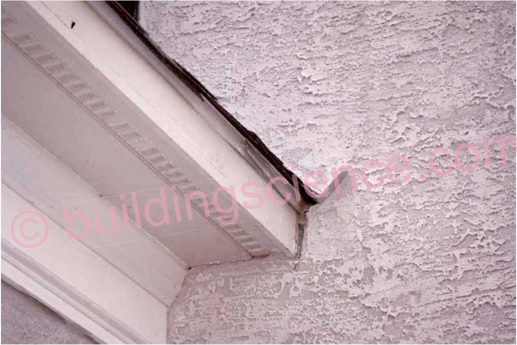
Photograph 39: Kick Out Flashing
