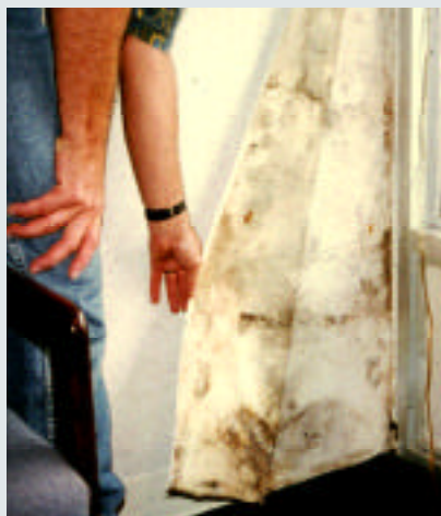
Mold growth behind vinyl wall covering.
