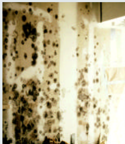
Mold growth on vinyl wall covering.
