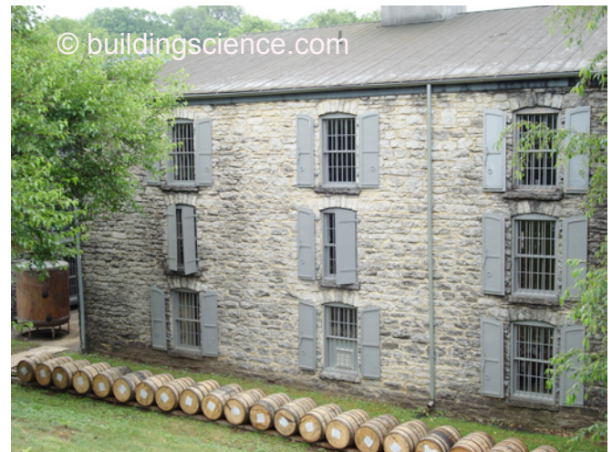
Photograph 5: High Mass Warehouse —Metal roof over timber deck, stone walls, dirt crawlspace, cross ventilation and stack ventilation. The temperature of the ground and the thermal resistance and thermal mass of the walls moderate the temperature swings within the building. The metal roof is cooler than asphalt shingles or a built up roof.
