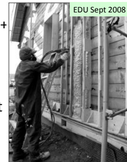
Figure 2. Dimension lumber and plywood trusses screwed to the sheathing on sixteen-inch centers provide adequate insulation space and a nailing base for finish siding.
